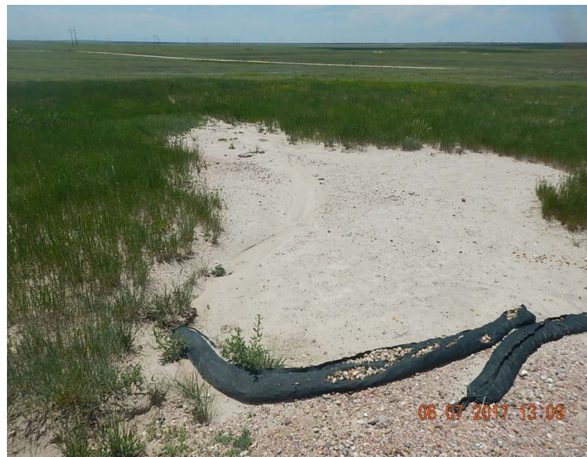
Photo 2: Stormwater erosion on S side of location, failure of wattle BMP.
