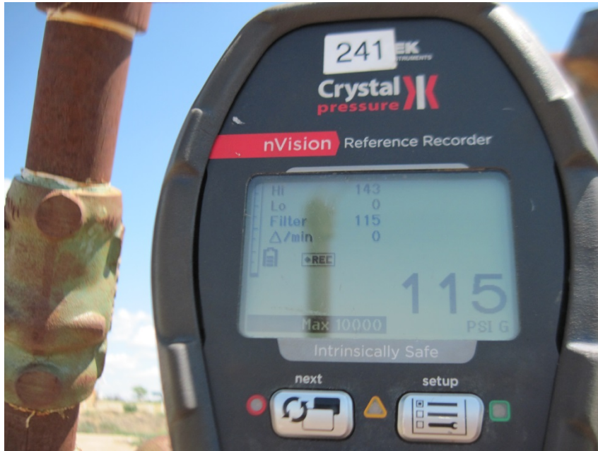
VRU SUCTION LINE
