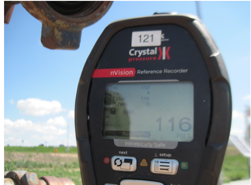
VRU DISCHARGE LINE
