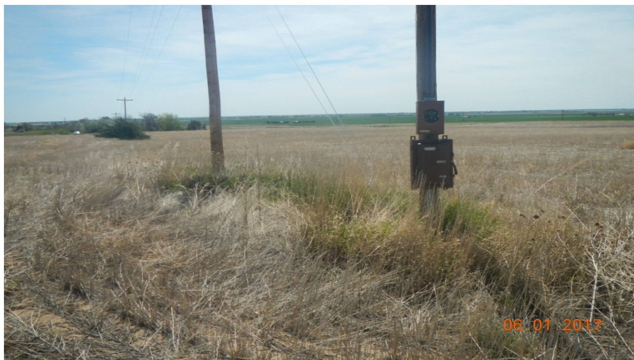
photo 4: The electric powerline utility terminates at the location.
