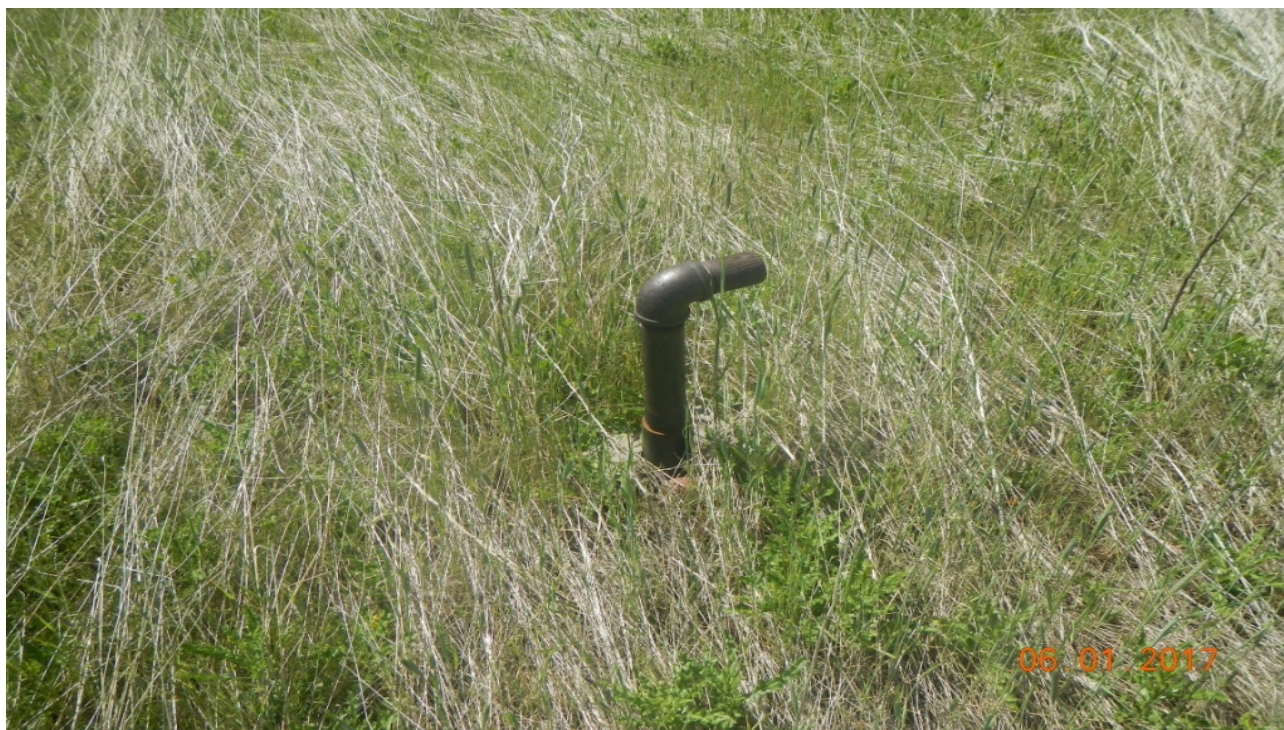
photo 4: An unknown pipe riser remains at the location. Lat/Long:39.78410,-104.36549.
