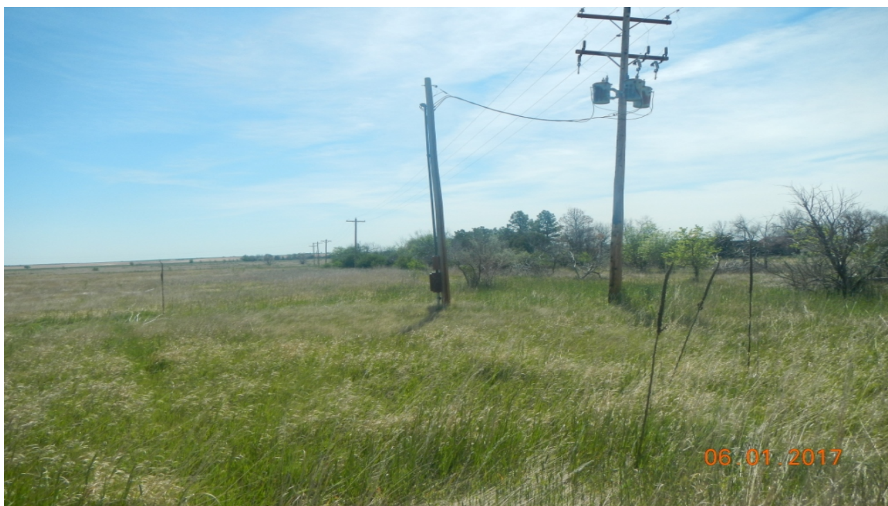
photo 4: The electric powerline utility remains at the location.
