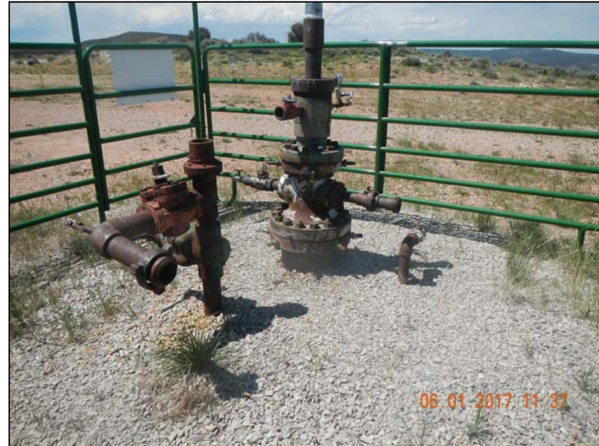
Photo 2. 1 – 2” and 1 – 3” steel riser at wellhead.
