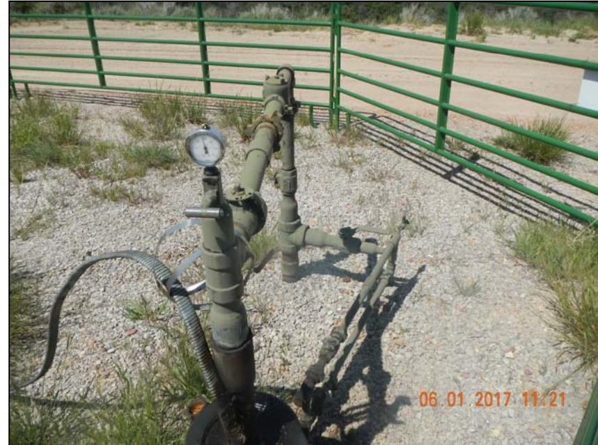
Photo 2. 1 - 2" steel riser at wellhead.
