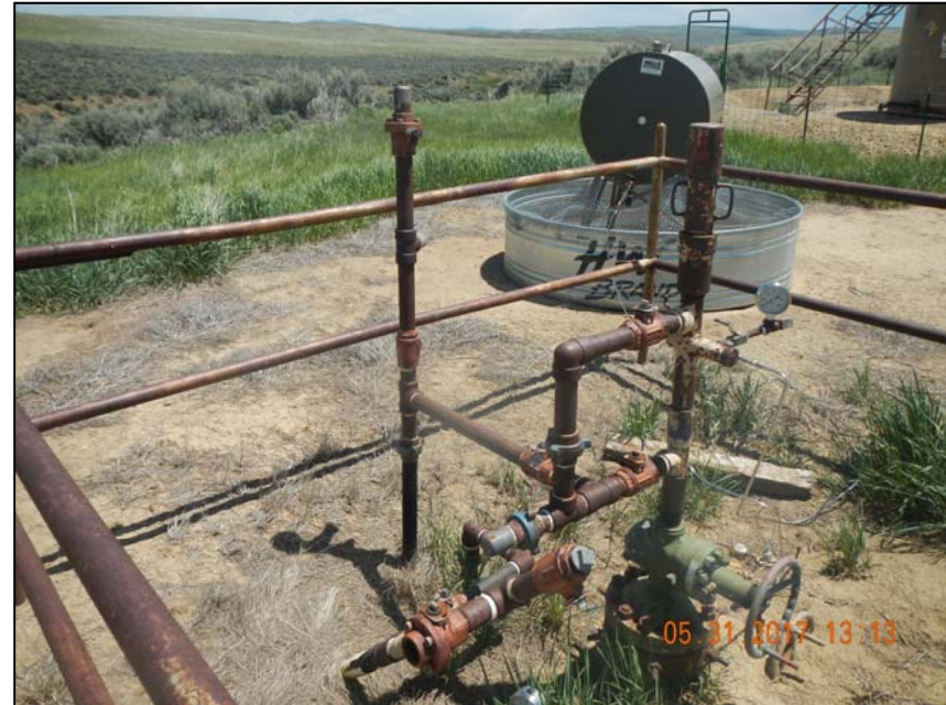
Photo 2. 3 - 2" steel riser at wellhead.
