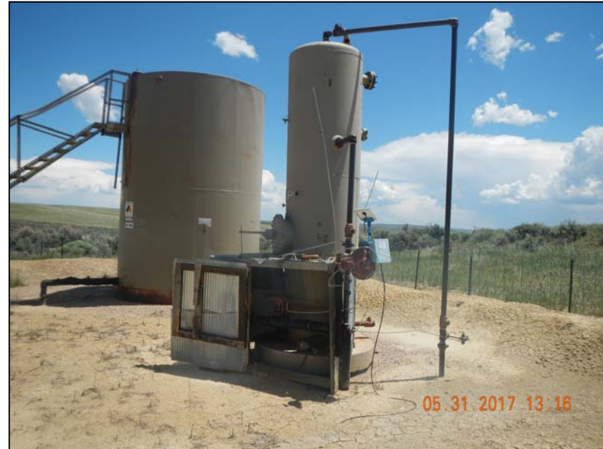
Photo 4. Risers at separator and tank.
