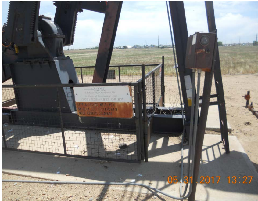
Sign washed out
