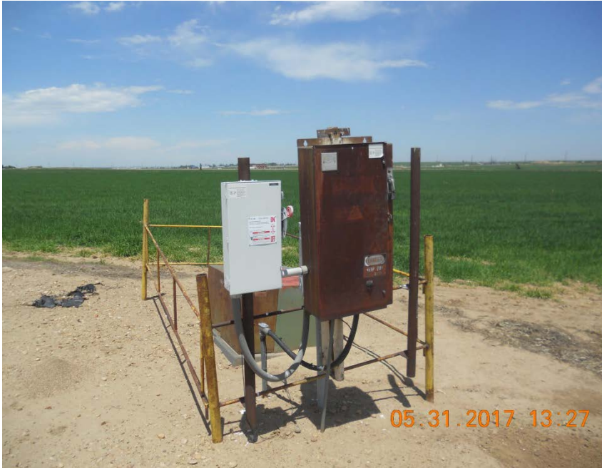
Electrical equipment east of pumpjack
