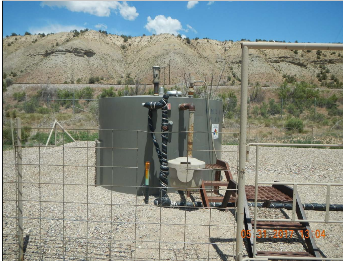
Tank Battery with a n used 2" riser painted orange.
