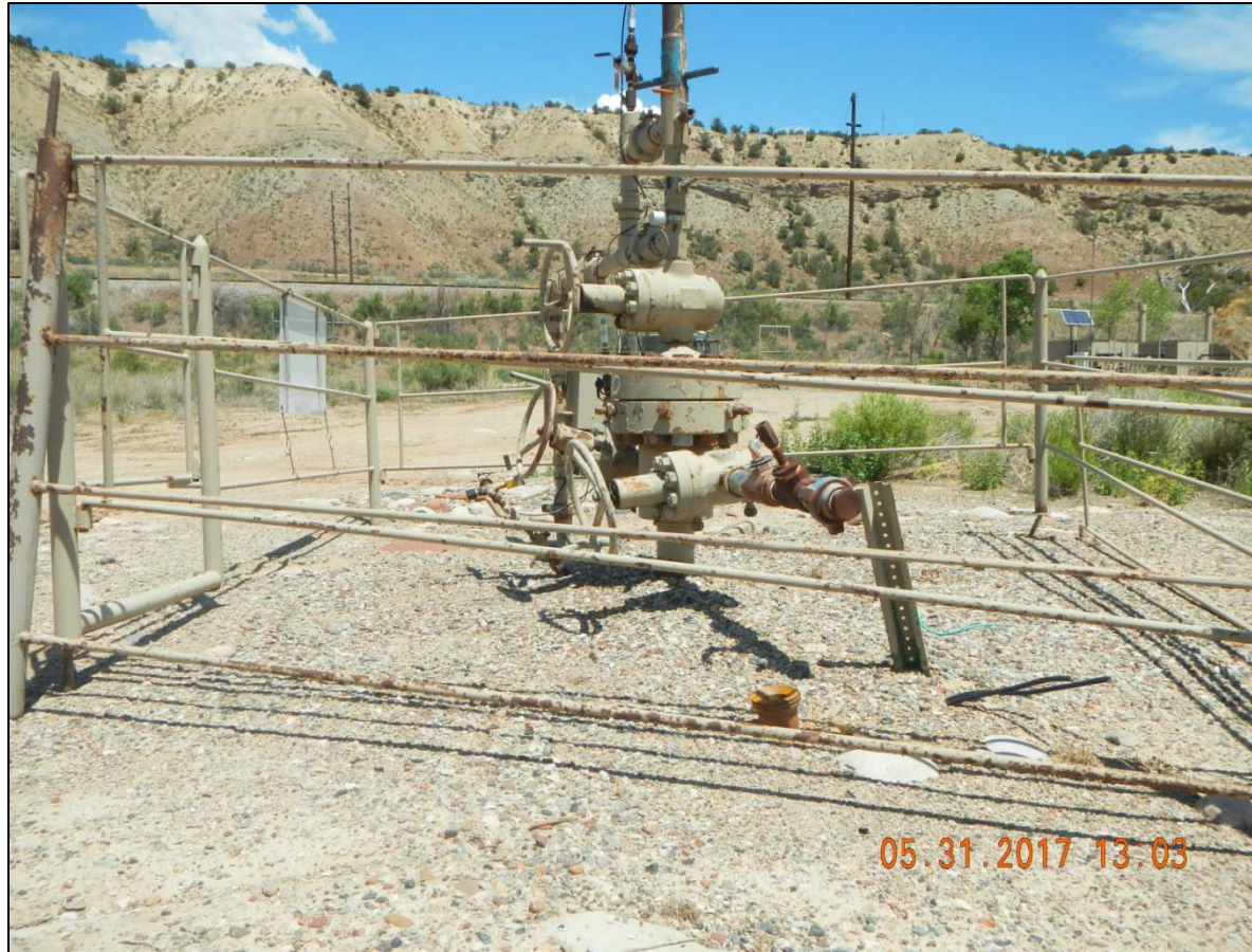
Unused riser painted orange at well head GM 24-1
