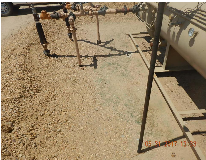
Photo 3: Risers at separator
