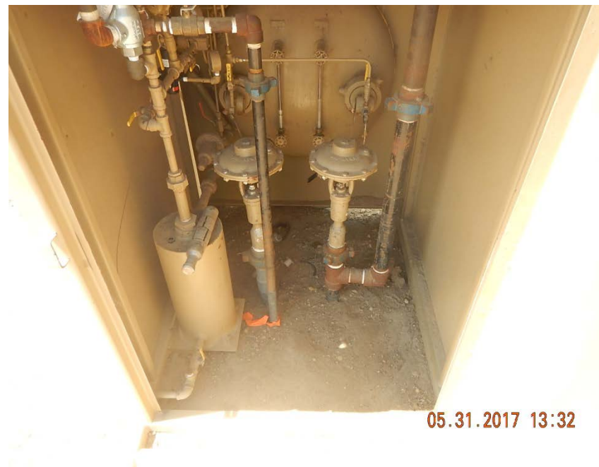
Photo 4: Risers in separator
