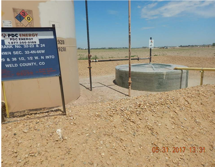
Photo 5: Risers at tank battery
