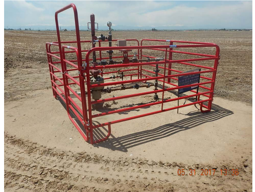
Photo 2: Risers at wellhead
