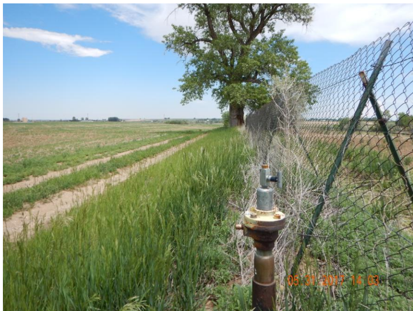
Photo 3. Riser #2 taken northeast of the well location.
