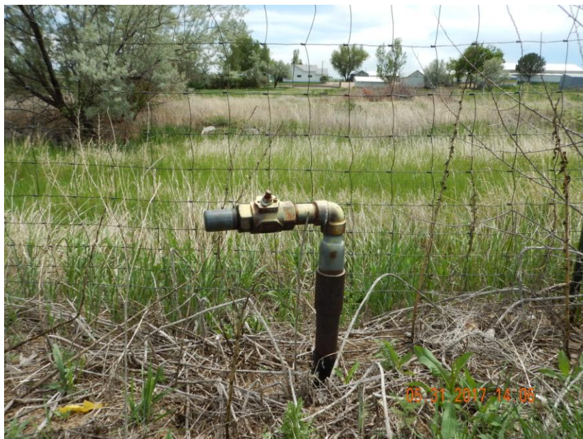
Photo 5. Riser #3 taken northeast of the well location.
