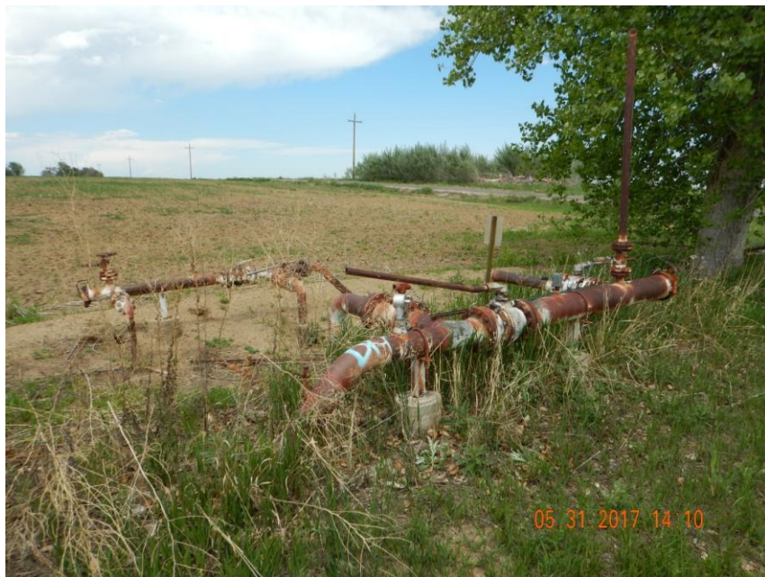
Photo 7. Riser #4 taken northeast of the well location. Not certain whether or not this is associated with the State #2-36 location or not.
