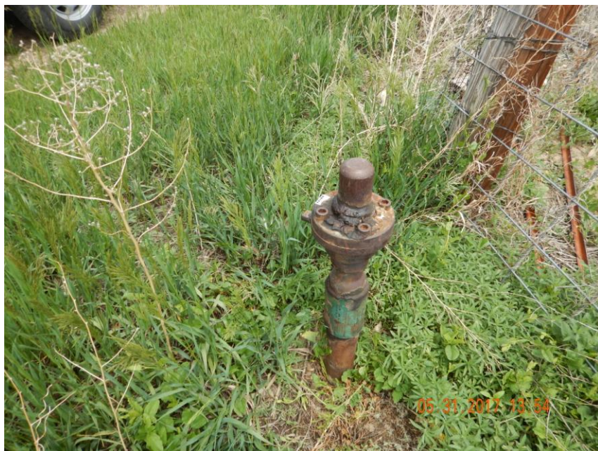
Photo 1. Riser #1 taken north of the well location.
