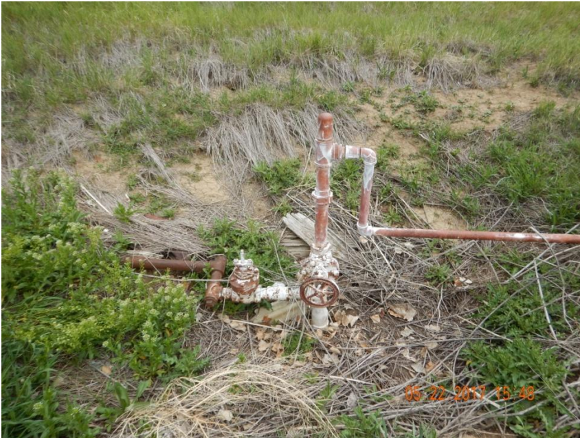
Photo 1. Photo taken from the depressed area, facing North. A partially buried flowline from this setup appears to be connected to the house illustrated in the previous aerial photo.
