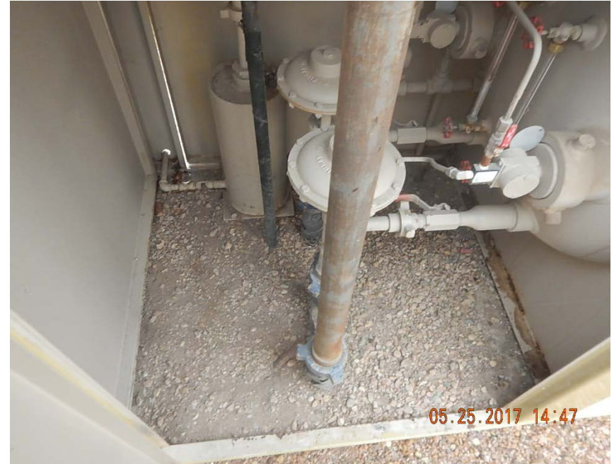
Photo 6: Risers in separators
