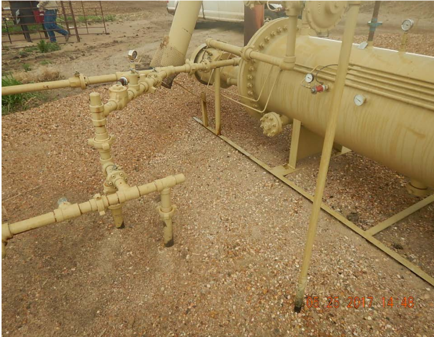
Photo 5: Risers at Separator
