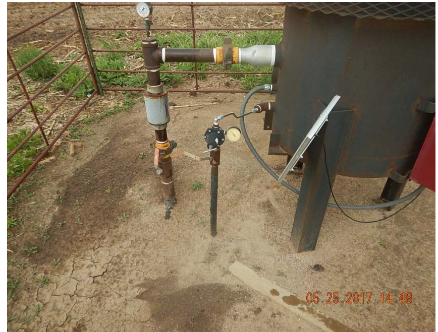
Photo 4: Risers at ECD
