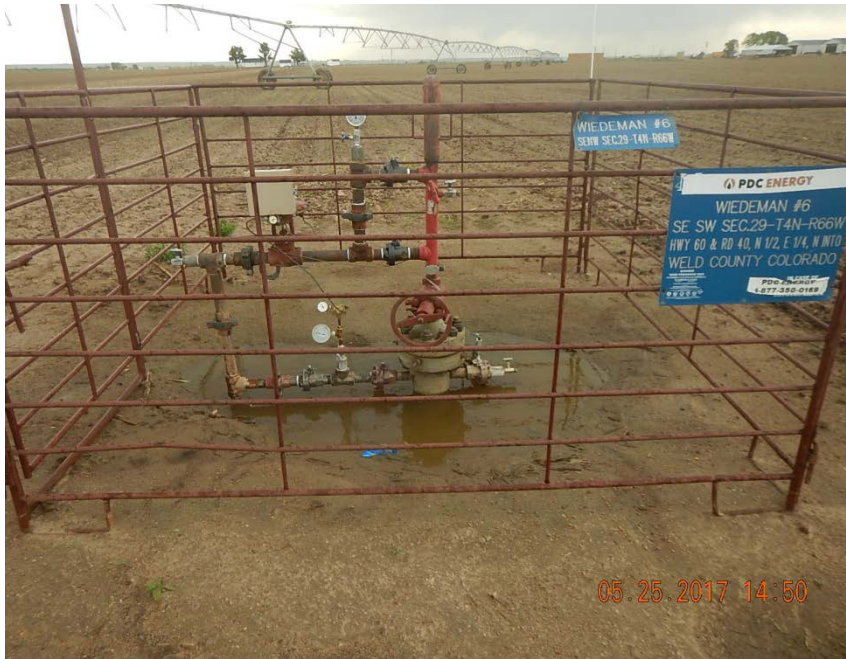
Photo 3: Risers at wellhead
