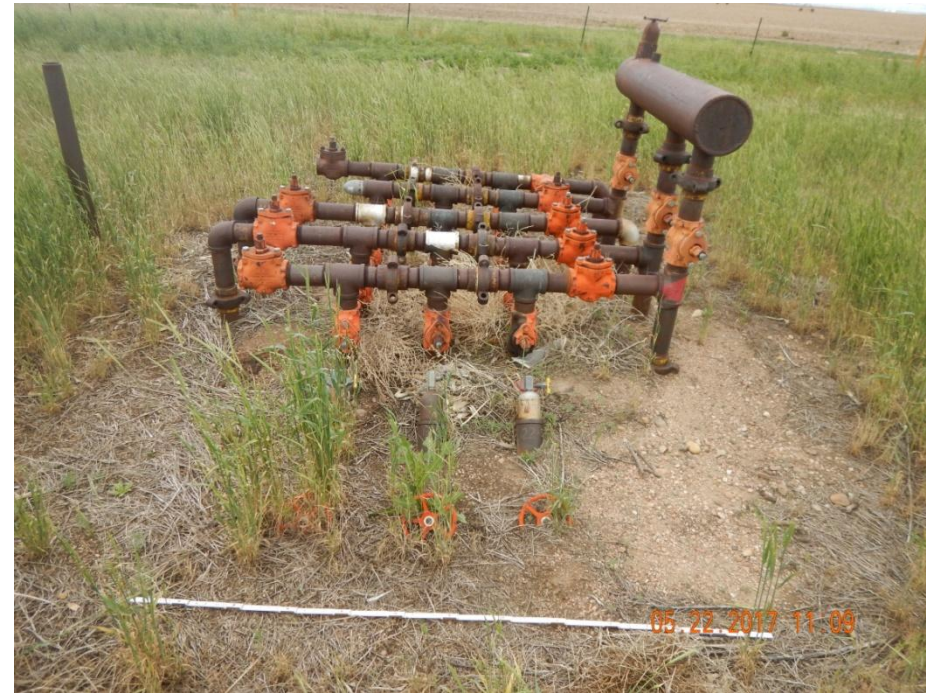
Photo 22: Photo of “~4 inch multi line w/ ~4 inch risers x2”
