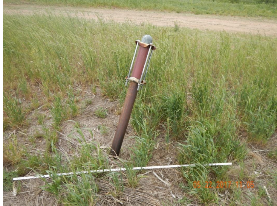
Photo 5: Photo of “~4 inch riser @ground” / “~4 inch riser”
