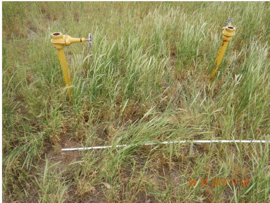
Photo 6: Photo of “~3 inch x2, yellow”
