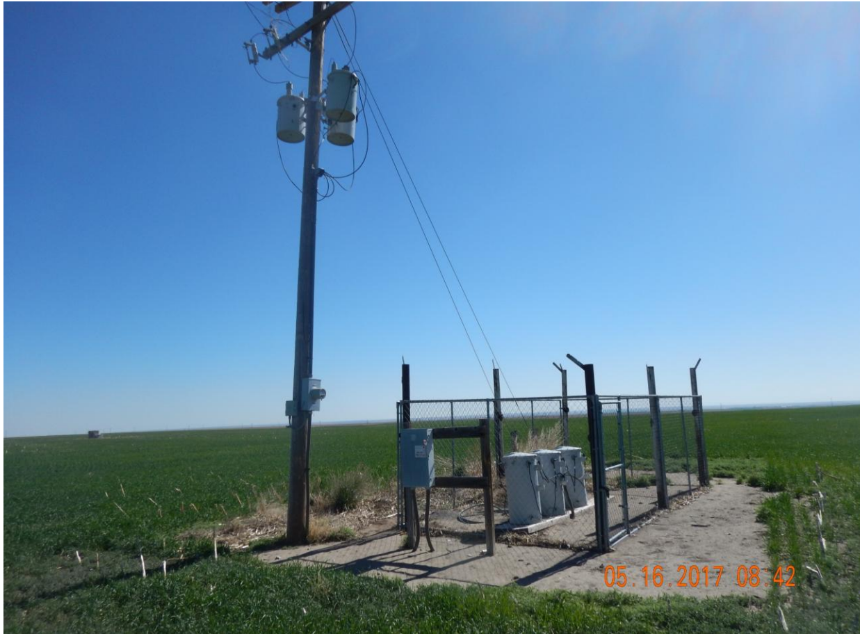
Photo 6: Photo taken to the north end of the location. Photo shows utilities that belong to the Flessner 1-A (121-09201) well directly to the east.
