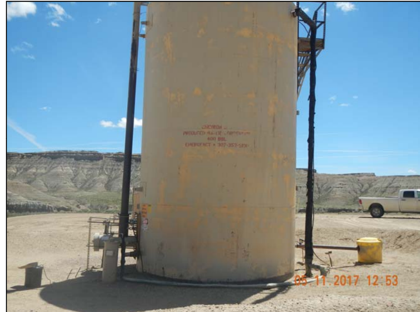
Photo 3. Chevron still on tanks.
