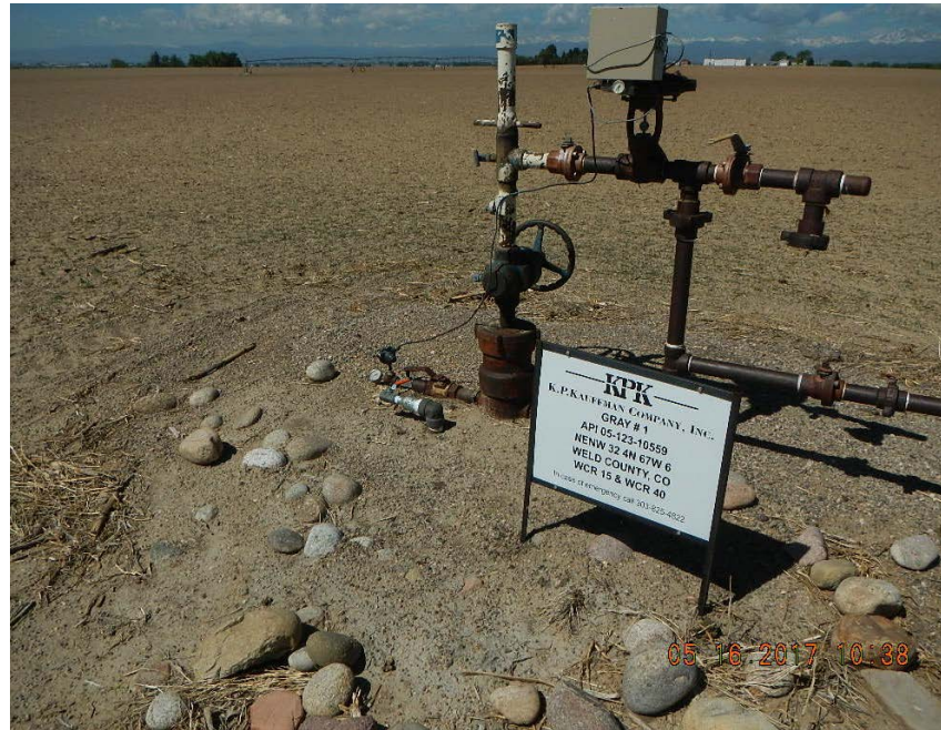
Wellhead sign and Bradenhead valve
