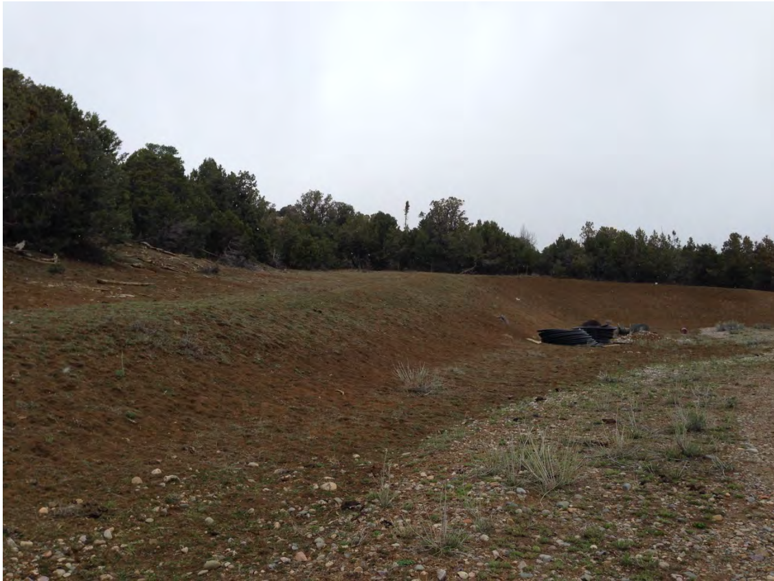
Photo 4 - Crader 3-3 cut wall and upper diversion ditch. Materials to be removed. View to north.
