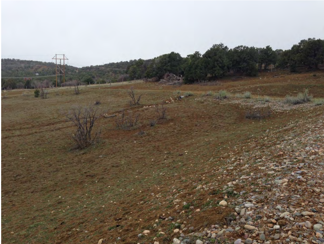
Photo 10 – Upper diversion ditch discharge south end. Note rills (to be mitigated) and grazing condition. View to south.
