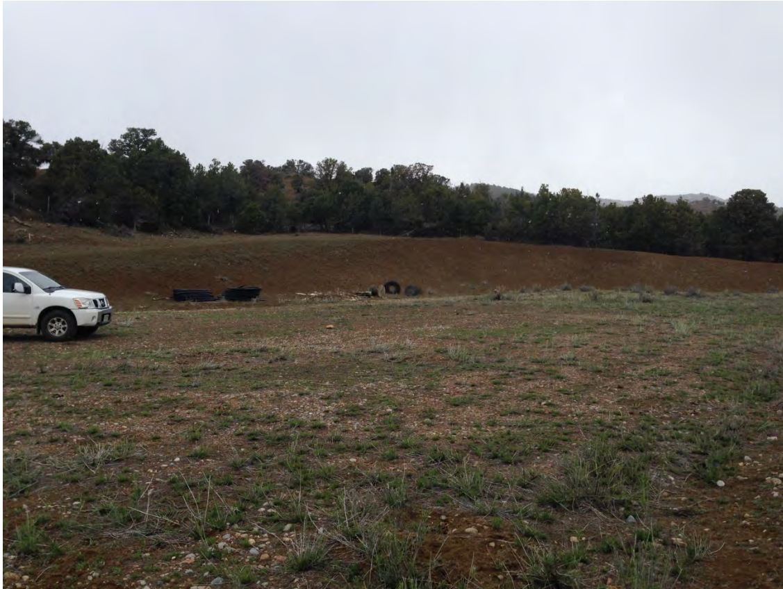
Photo 8 – Crader 3-3 pad and cut wall. Stored materials to be removed. View to northwest.
