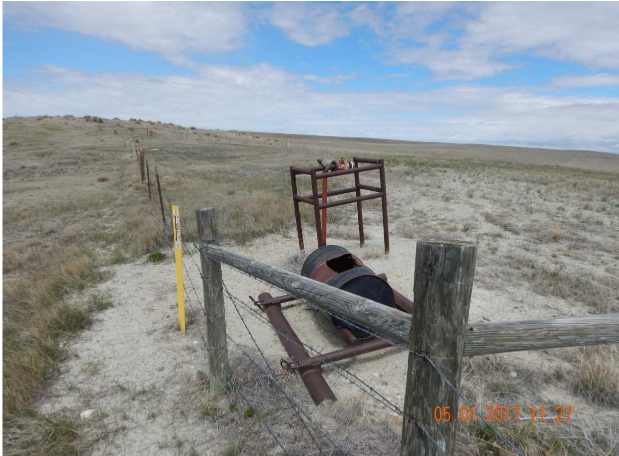
Photo 1: Photo taken from the south end of the location, facing west. Photo shows pipe riser and debris has not been removed from location.
