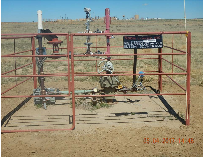
Photo 1: Wellhead, looking NW
