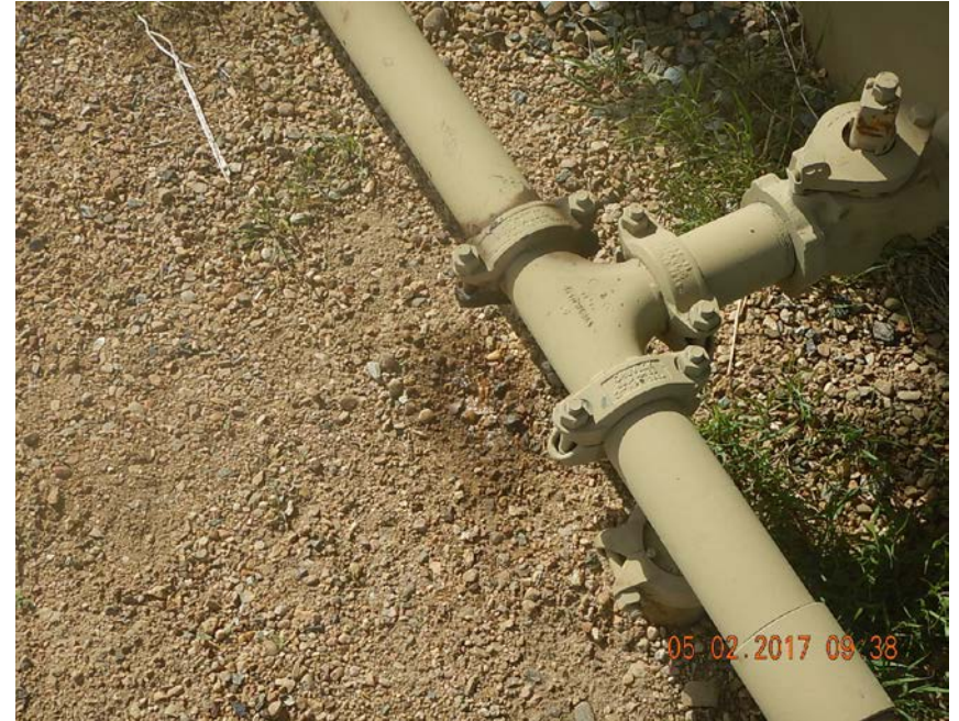
Photo 4: Stained soil removed, new stained soil at fitting.
