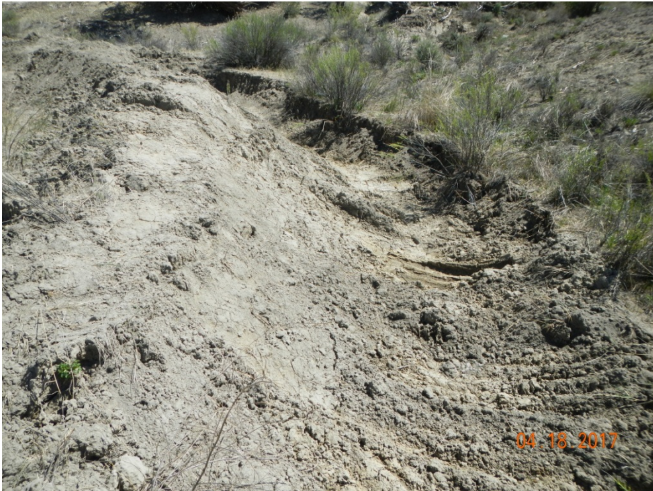
Photo 3: View of diversion channel that was recently graded. Soil is not stabilized and needs to be stabilized with erosion and sediment controls (i.e. vegetation and check dams).
