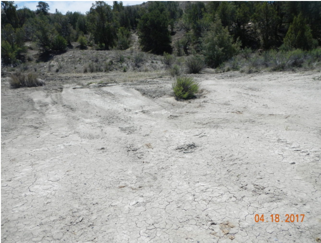
Photo 2: View of the southeastern portion of the working area where erosional channel is filled. Vegetation has been damaged and removed, and bare areas need revegetation.
