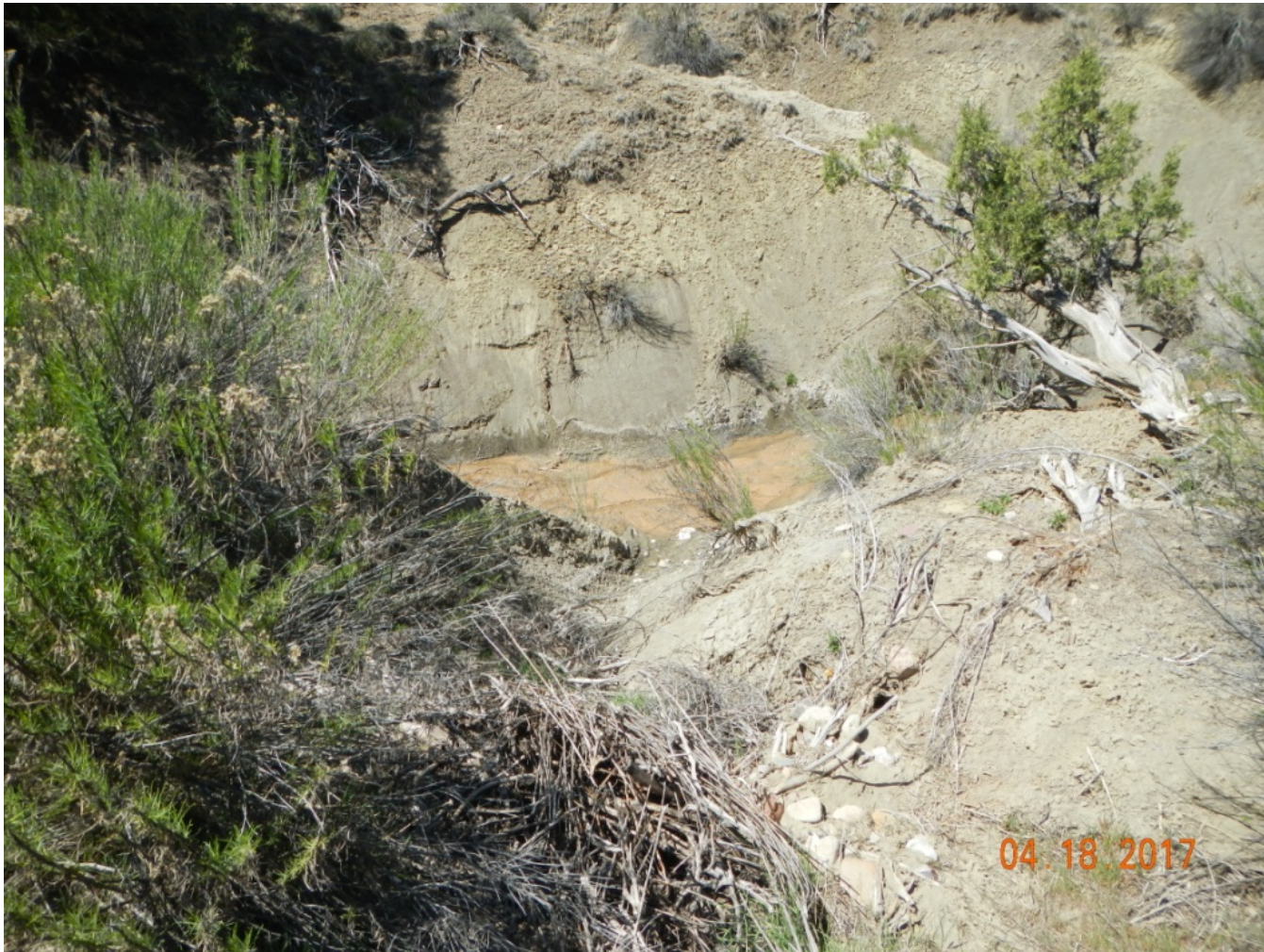
Photo 7: View of area where stormwater flows from the roadside drainage in Photo 6 into a stream, and is eroding the bank.
