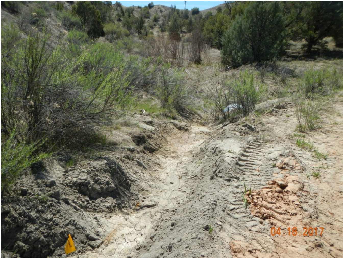
Photo 9: View of area where stormwater flows from the roadside ditch in Photo 8 into a stream and is eroding the bank. Soils are exposed and no erosion or sediment controls are in place.
