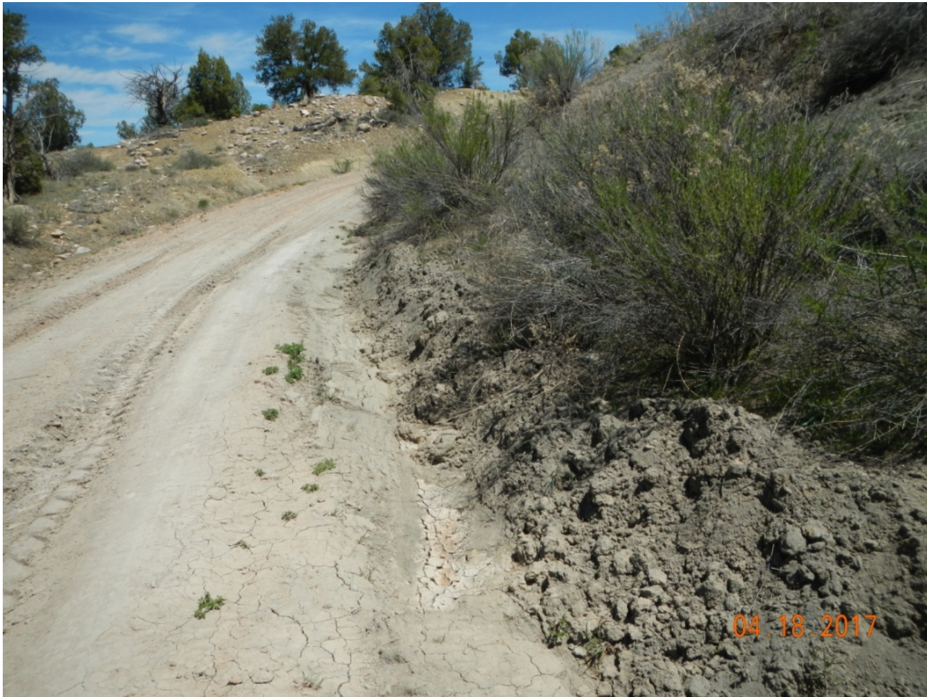
Photo 8: View of drainage along southern edge of access that was recently scraped. Soils are exposed and no sediment controls are in place.
