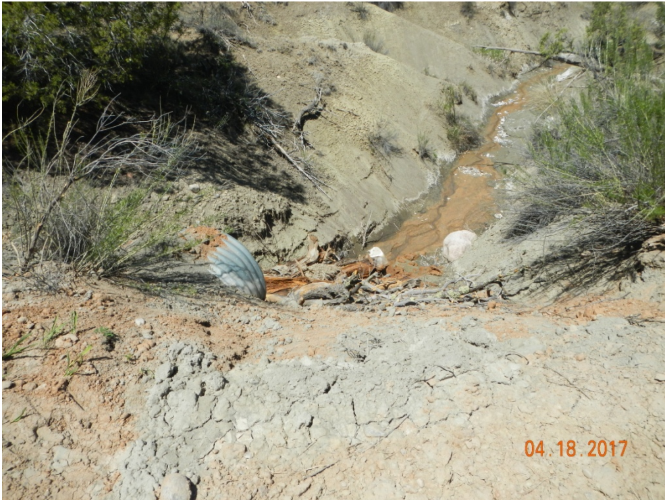
Photo 5: View of area at culvert along access road where erosional channel was filled with soil but is not stabilized.
