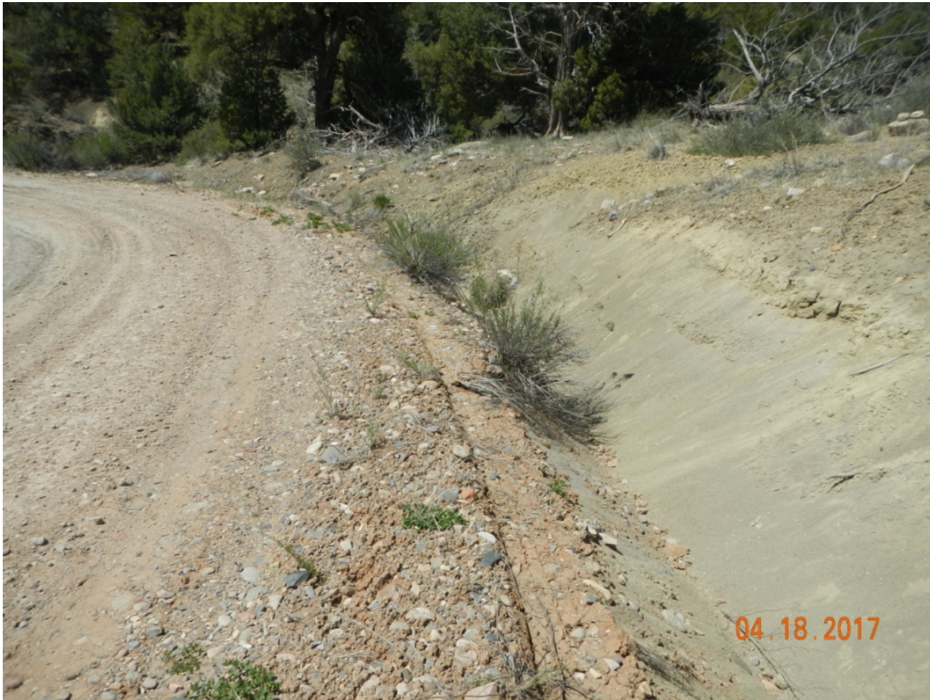
Photo 6: View of drainage along northern edge of access that was recently scraped. Soils are exposed and no sediment controls are in place.
