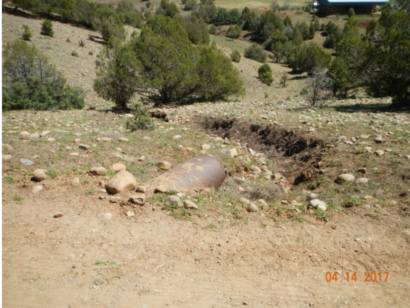
Photo 5: View of erosional channel at culvert along access. Erosion is approximately 2 feet deep and 3 feet wide. Needs to be stabilized.
