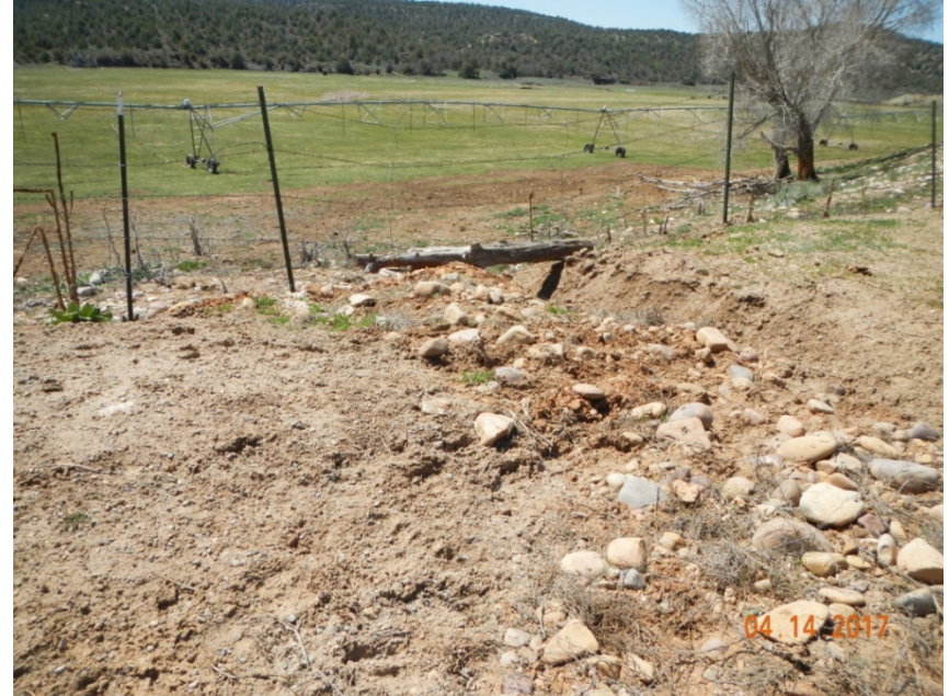
Photo 4: View of erosional channel forming within the southern portion of the project area.
