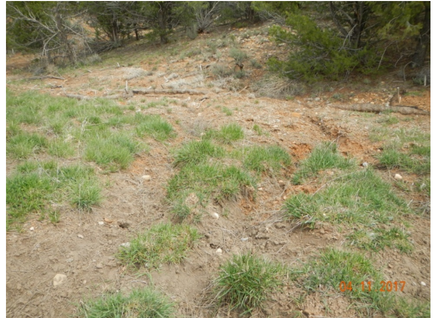
Photo 4: View of erosion and failed stormwater controls within the eastern portion of the project area.
