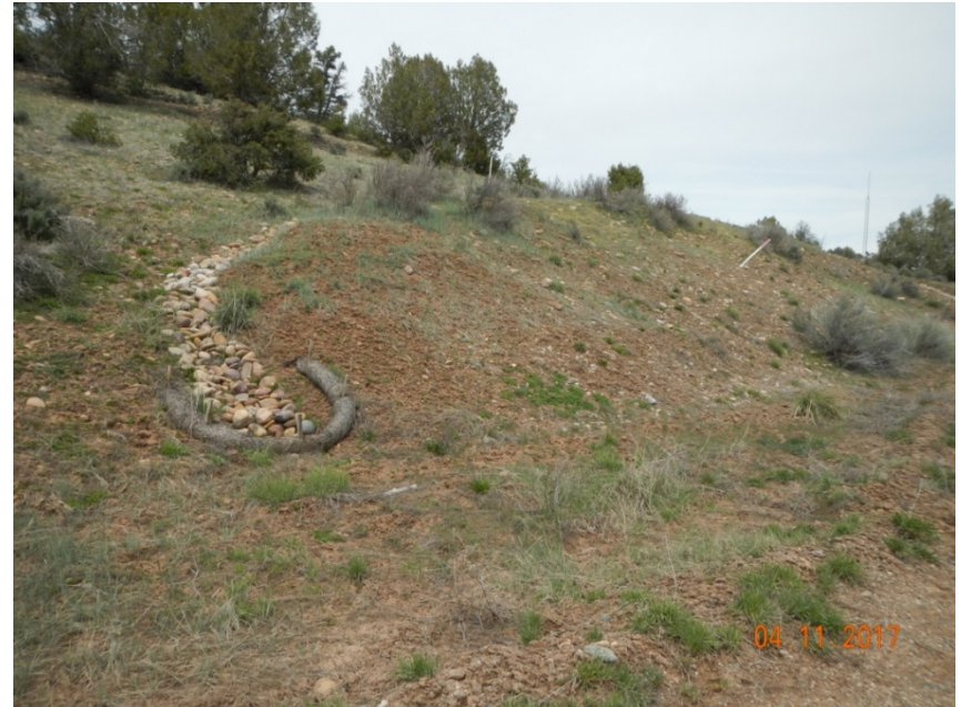
Photo 4: View of stormwater controls in the southwestern portion of the project area.
