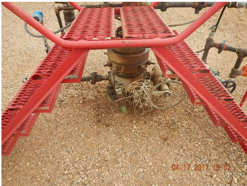
Photo 3: Stained soil at wellhead
