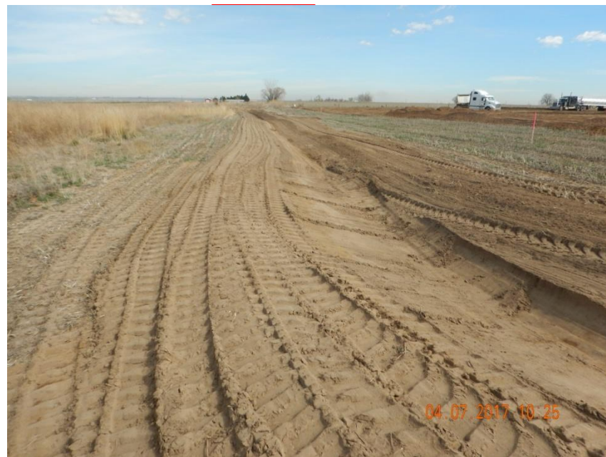
Photo 6. Photo taken from the southwest location, facing North. Ditch and berm BMP installed around the perimeter of location. Also, location is dominated by sandy soils so a tackifier is recommended to stabilize all disturbed areas to control for wind erosion.
