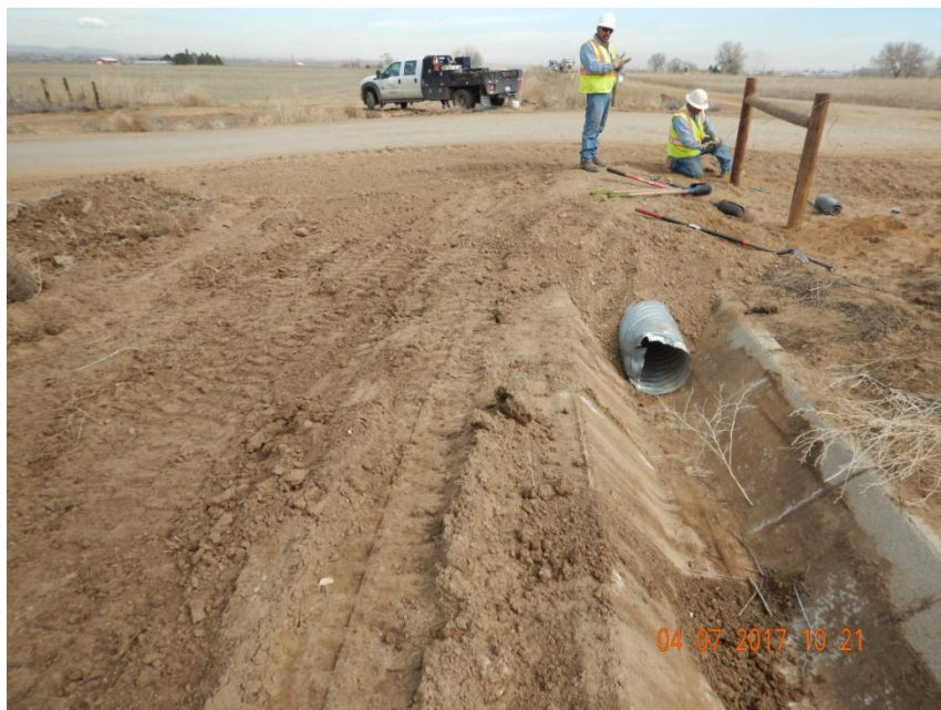
Photo 1. Photo taken from the entrance of location, facing North. Culvert installed in conjunction with the existing irrigation ditch. Operator shall ensure that sediment is not discharged into the ditch and ensure soil material is stabilized around the culvert.
