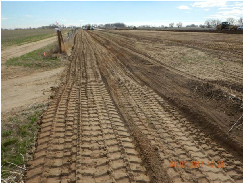
Photo 9. Photo taken from the northern location, facing East. Ditch and berm BMP installed around the perimeter of location. Also, location is dominated by sandy soils so a tackifier is recommended to stabilize all disturbed areas to control for wind erosion.
