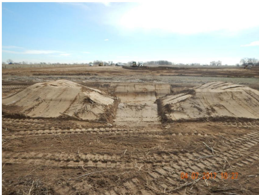
Photo 7. Photo taken from the western location, facing East. Sediment trap installed and IN-PROCESS of being completed (i.e., outlet still needs to be stabilized). Also, location is dominated by sandy soils so a tackifier is recommended to stabilize all disturbed areas to control for wind erosion.
