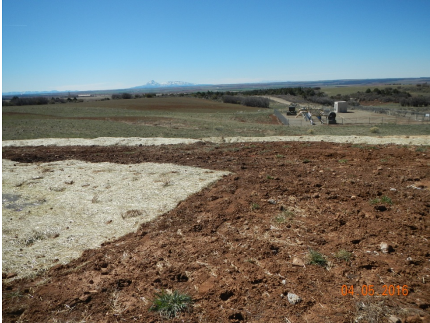
Photo 5: View of stormwater controls newly installed within the southern portion of the project area. Appear to be functioning at this time. Area is recently seeded.
