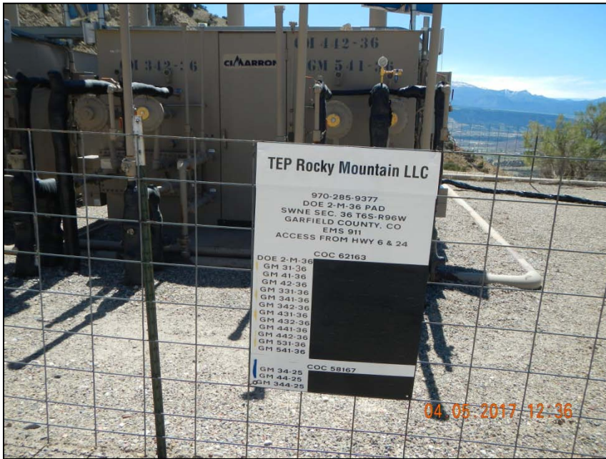
Battery sign at separators
