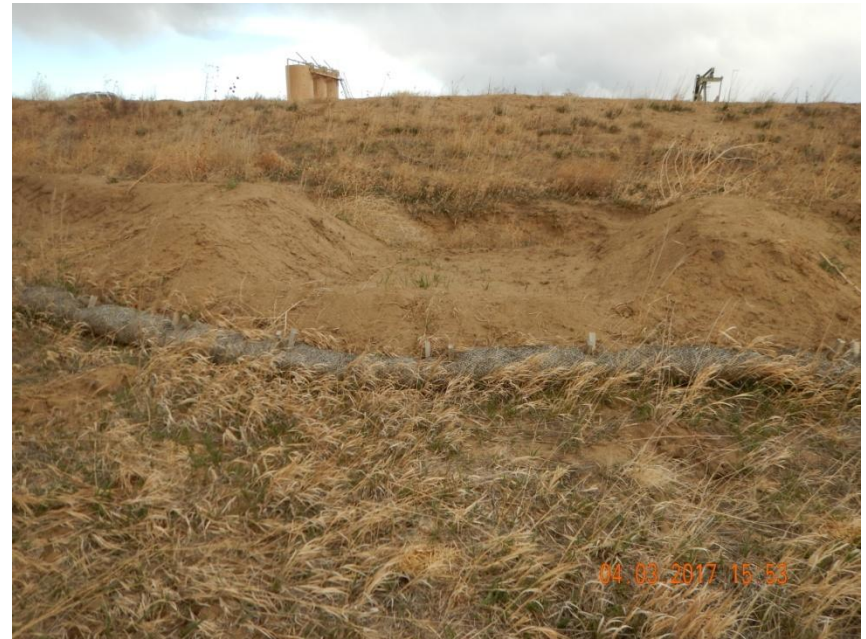
Photo 4. Photo taken from the southern sediment trap along the western location, facing East. Minor repairs were made to the sediment trap which may be insufficient to prevent sediment laden stormwater runoff from leaving location.
