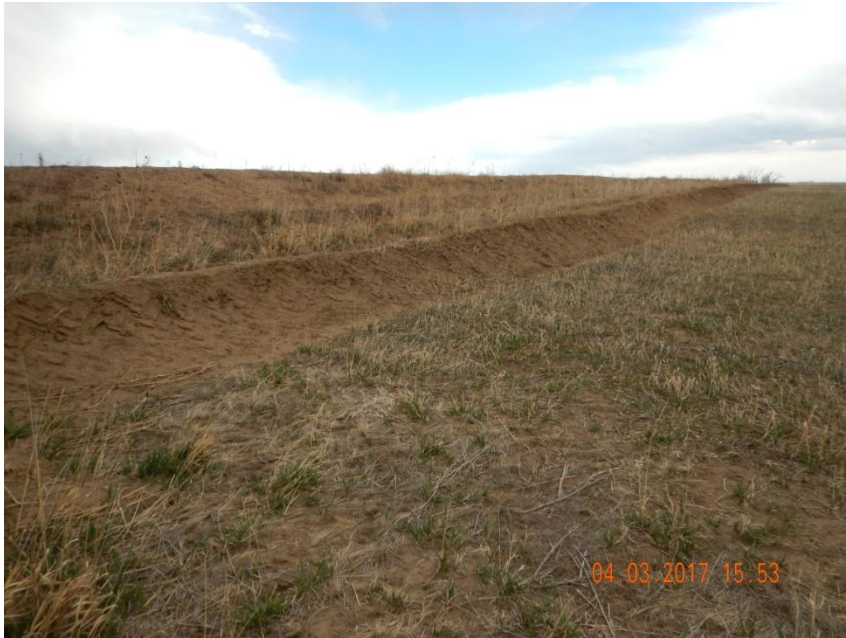
Photo 5. Photo taken of the western location, facing Southeast. Berm BMP has been repaired and built up higher.
