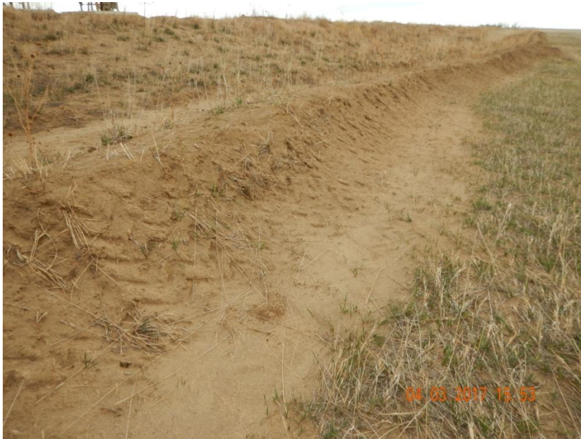
Photo 3. Photo taken of the northwestern location, facing South. Berm BMP has been repaired and built up higher.
