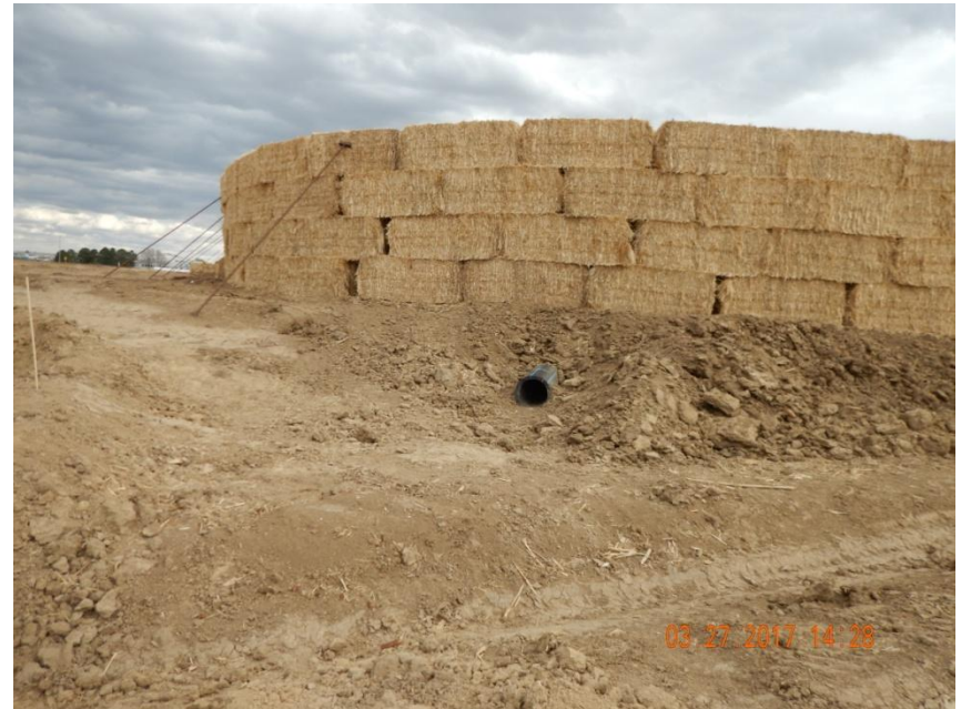
Photo 8. Photo taken from the northwest location, facing Southeast. Culvert has been installed directing stormwater runoff from the production area to the northwest sediment trap.
