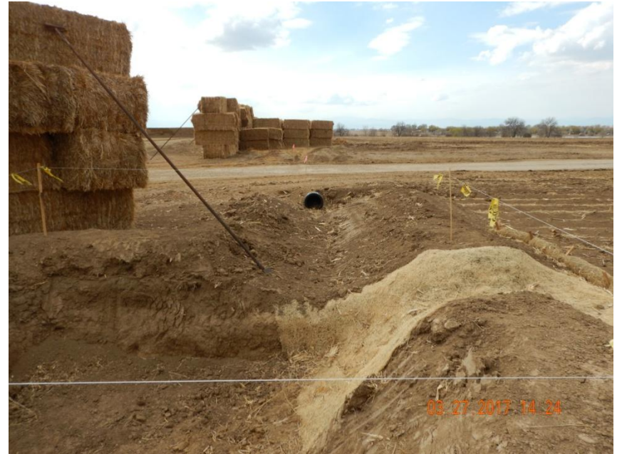
Photo 4. Photo taken from the northeast location, facing West. Culvert installed in conjunction with the ditch and berm BMP that is directed to the sediment trap.
