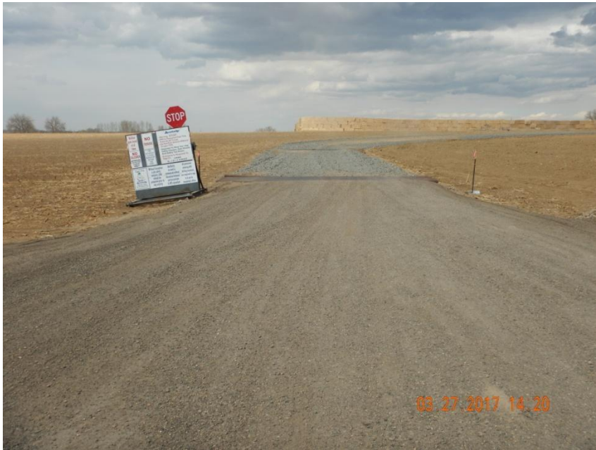
Photo 1. Photo taken from the entrance of location, facing North. Vehicle tracking pad installed and appears to be properly functioning.
