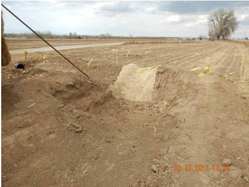
Photo 3. Photo taken from the northeast location, facing North. Sediment trap installed with outlet protection in the form of a blanket and wattle.
