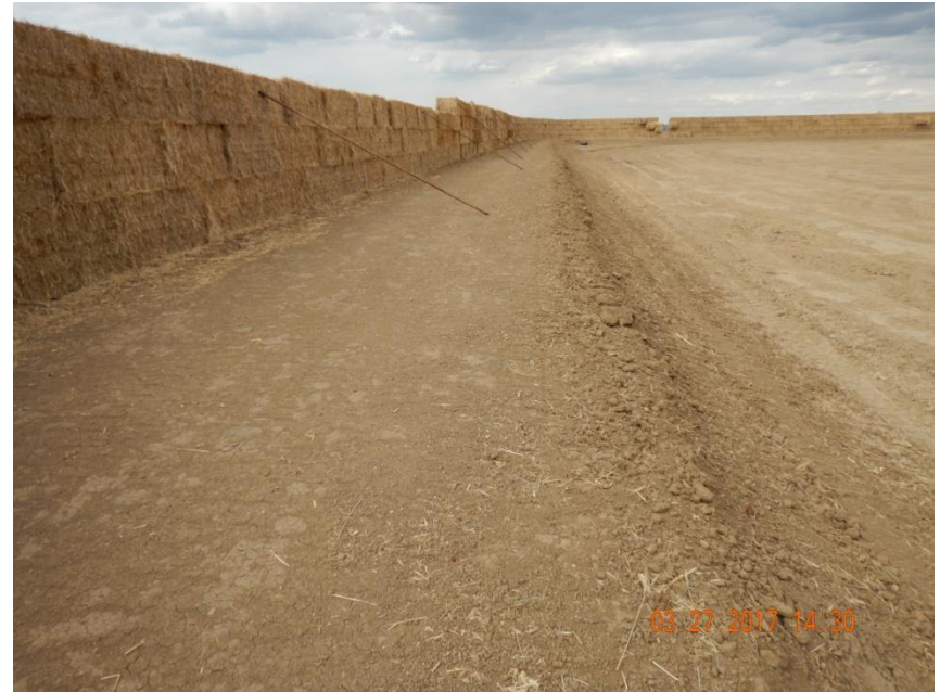
Photo 10. Photo taken from the western production location, facing North. Topsoil salvaged and stored along the northern and western perimeter of the production location.
