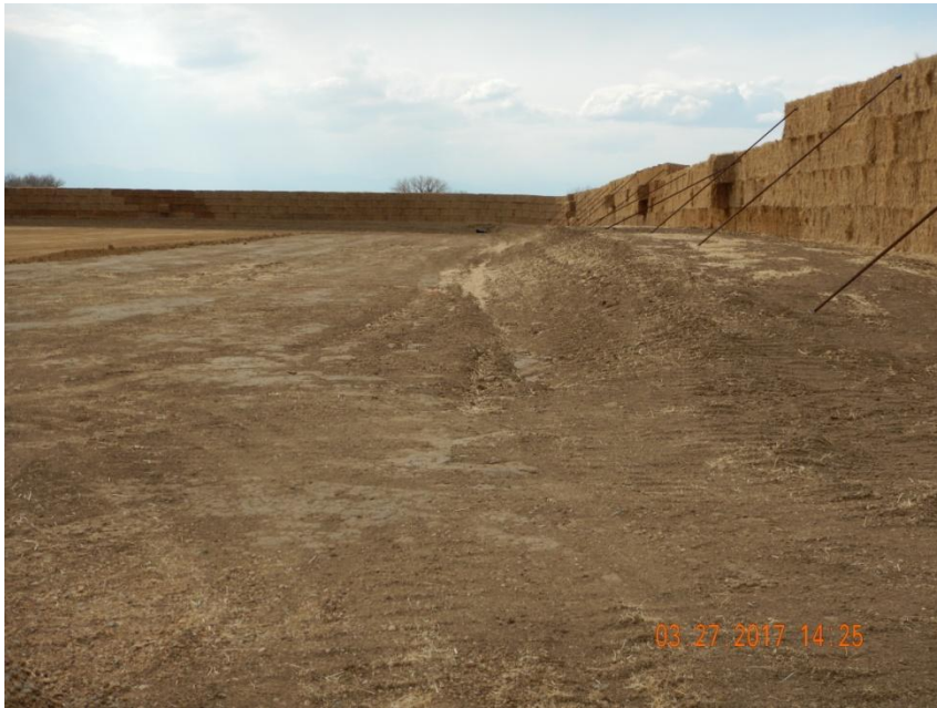
Photo 5. Photo taken from the northern production location, facing West. Topsoil salvaged and stored along the northern and western perimeter of the production location.
