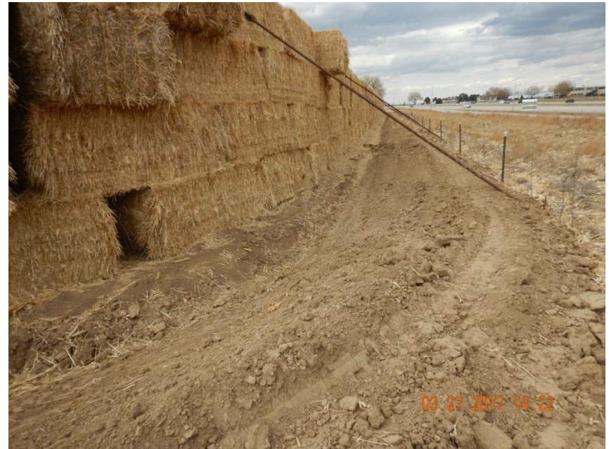
Photo 2. Photo taken from the southeast location, facing North. Ditch and berm BMP installed around perimeter of location.
