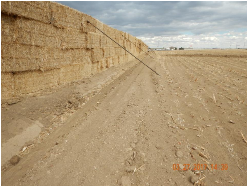
Photo 11. Photo taken from the southern location, facing East. Ditch and berm BMP installed around perimeter of location.
