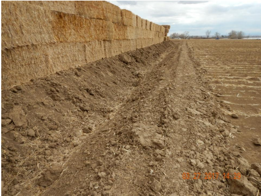
Photo 9. Photo taken from the western location, facing South. Ditch and berm BMP installed around perimeter of location.
