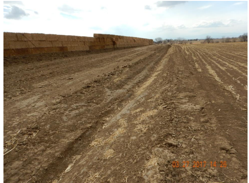
Photo 6. Photo taken from the northern location, facing West. Ditch and berm BMP installed around perimeter of location.
