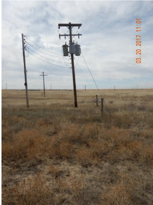
Photo 2: Photo taken from the north end of the location, facing south. Photo shows utility pole remaining on location
