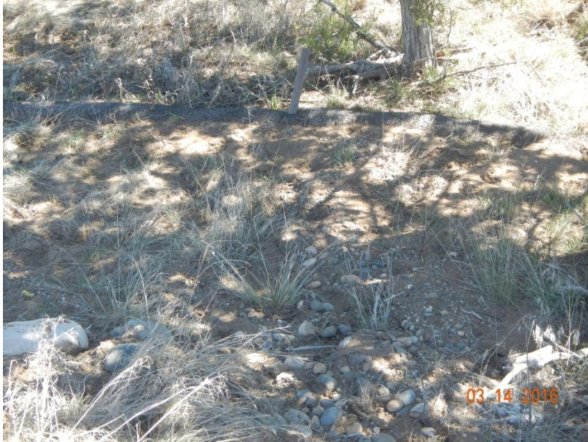
Photo 5: View of perimeter wattles that are full of sediment in the southeastern portion of the project area.
