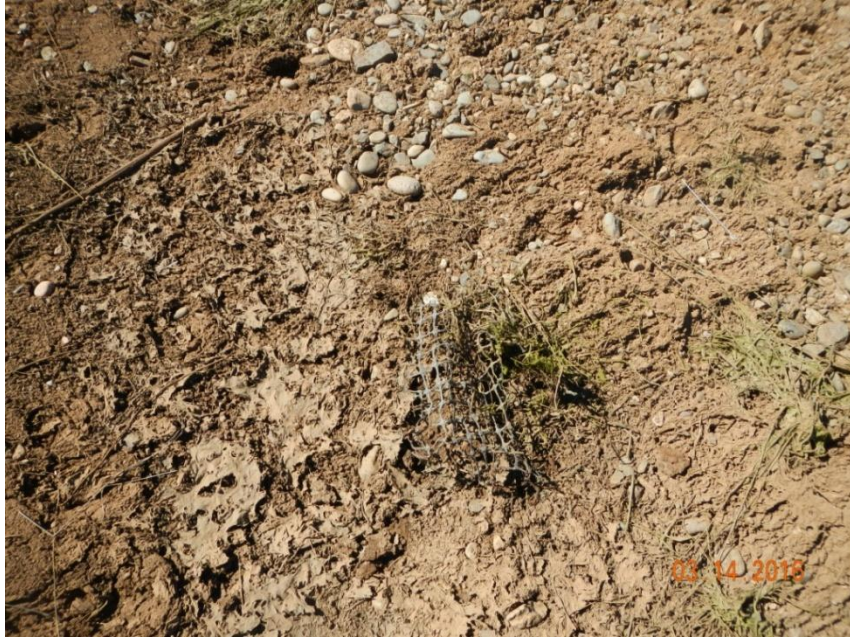
Photo 5: View of netting debris within the interim reclamation area. Additional pieces of netting and liner debris are scattered around the interim reclamation areas and should be cleaned up.
