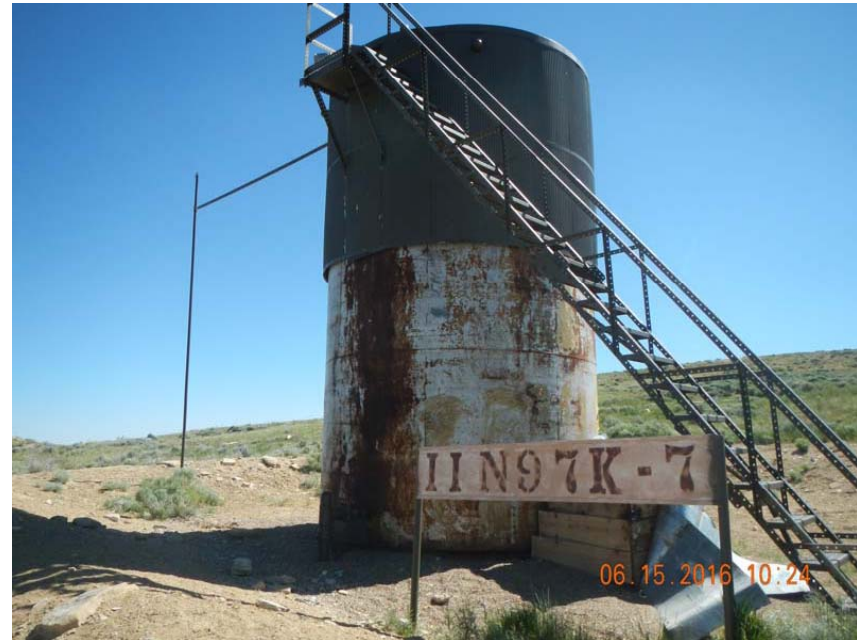
Photo 5. No tank label from 6/15/2016 inspection.
