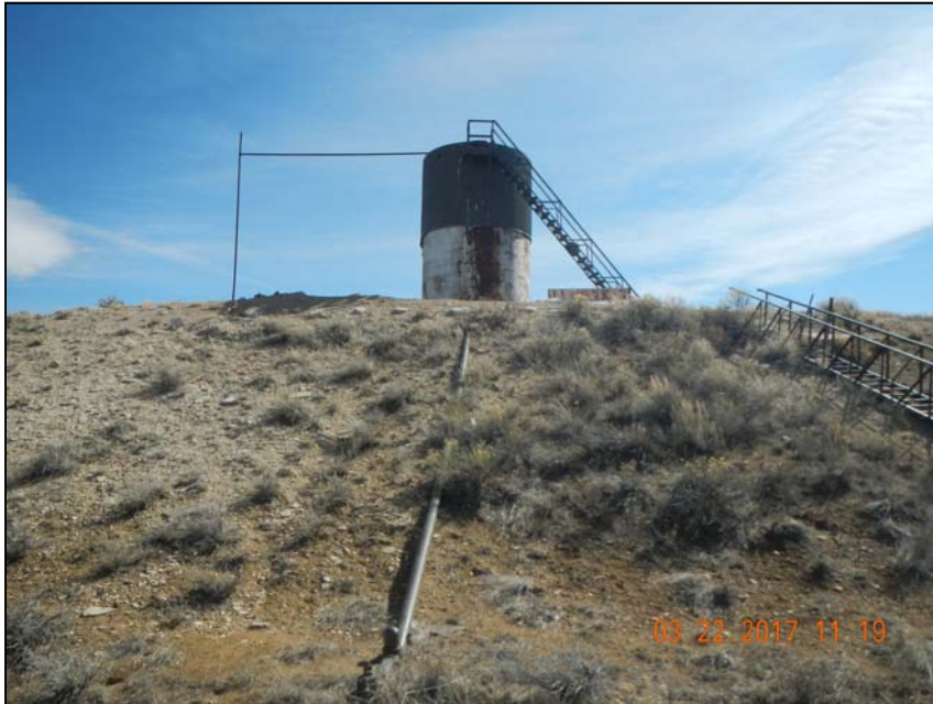
Photo 4. No tank label.
