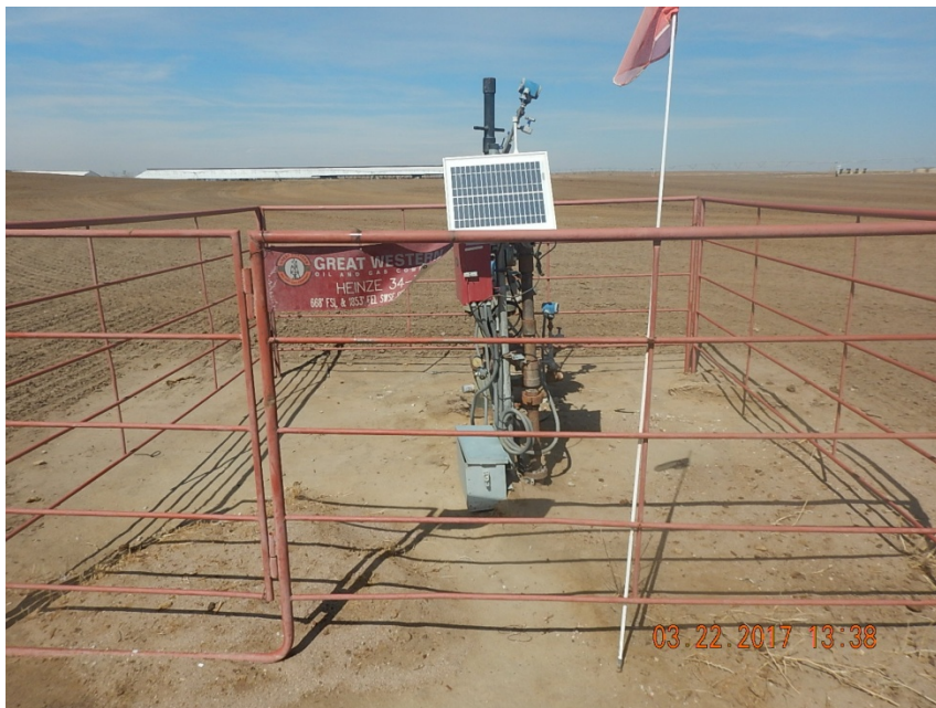
Photo 1: Wellhead, looking N
