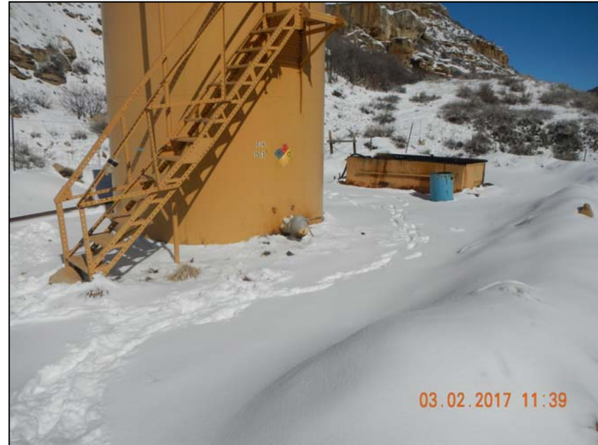
Photo 2. Incomplete tank label.
