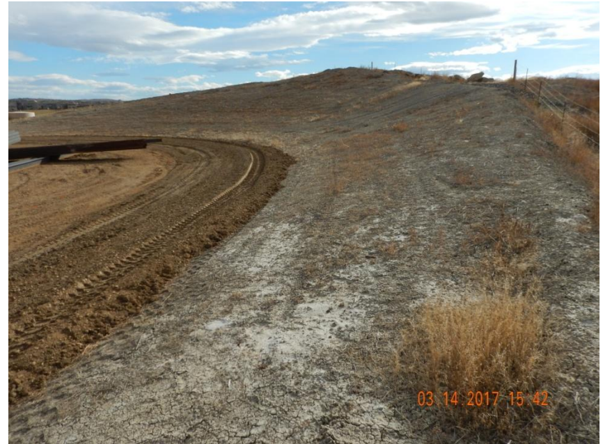
Photo 6. Photo taken from the southwestern location, facing South. The cut slope appears to be stabilized and BMPs have been installed on the uphill side- see following photos.
