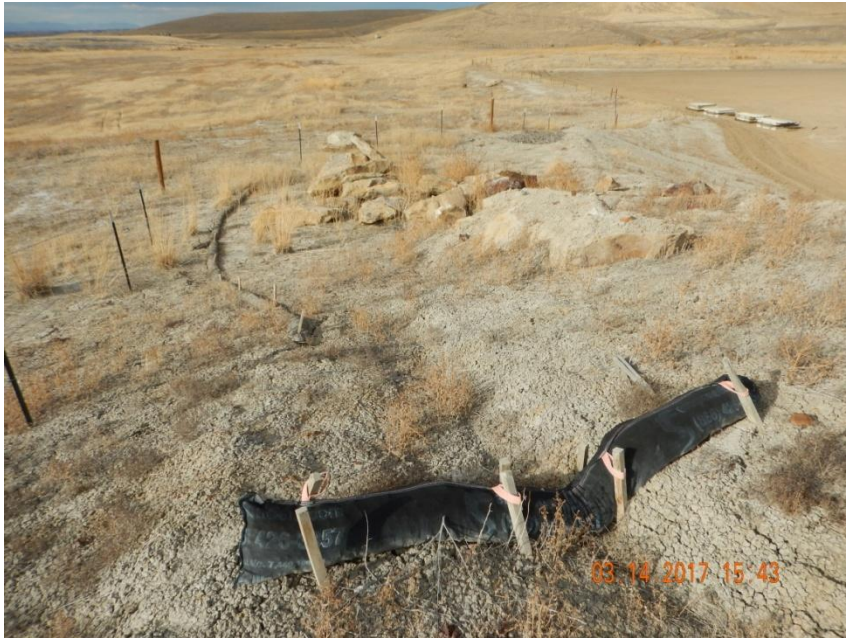
Photo 7. Photo taken from the southwestern location along the uphill side of the cut slope, facing North. Wattles have been installed in conjunction with the ditch BMP. Some of the straw wattles may need maintenance or repairs.
