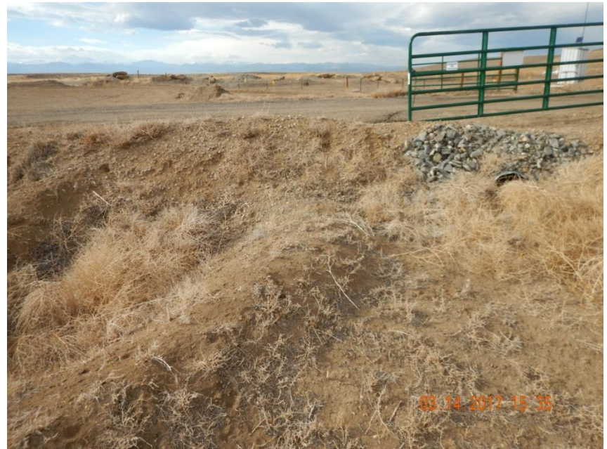
Photo 2. Photo taken from the well site entrance, facing North. Culvert has both inlet and outlet protection; however, the culvert doesn't appear to be directed to the ditch and berm BMP. May need to ensure culvert and ditch and berm BMP are connected to ensure containment of stormwater runoff.
