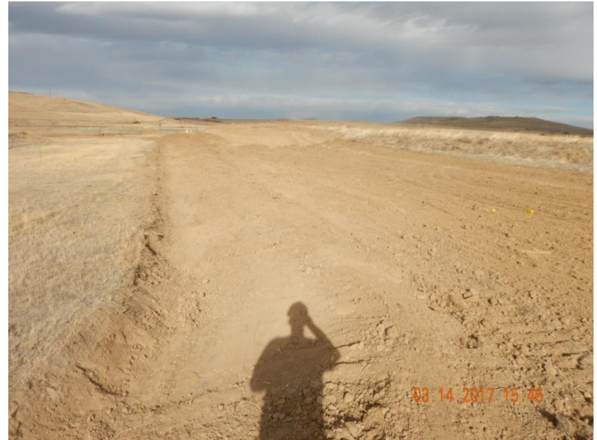
Photo 12. Photo taken from the eastern location, facing North. A ditch and berm BMP has been installed around the perimeter of the location.
