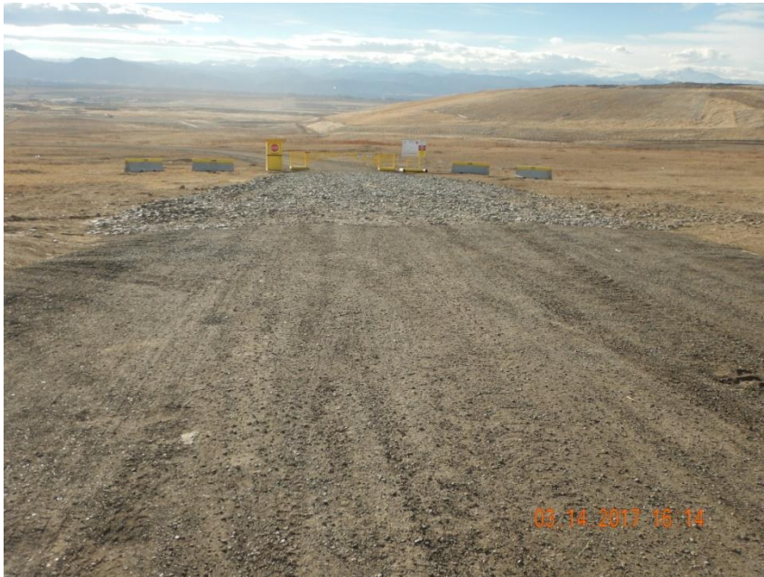
Photo 1. Photo taken from the entrance of location off Country Road 5, facing West. Vehicle tracking pad installed.
