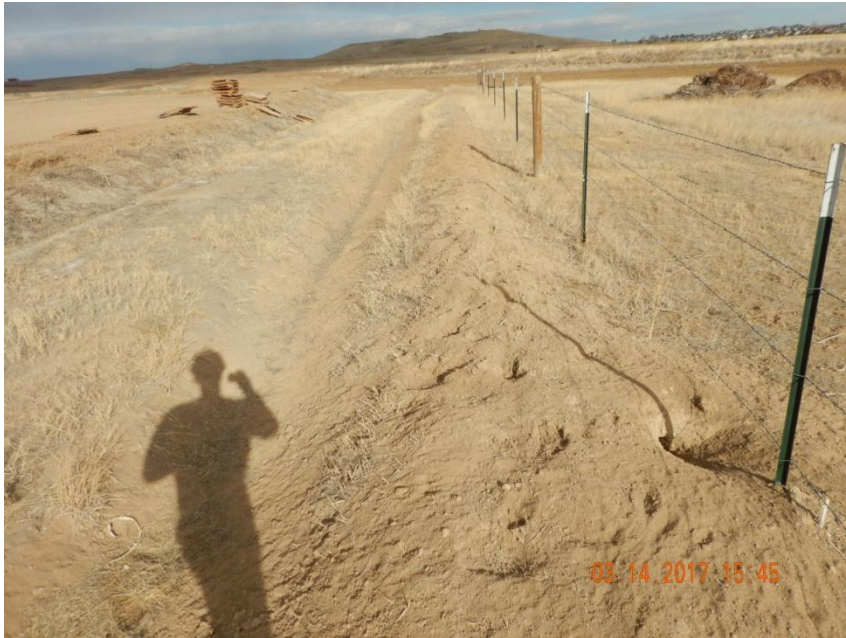
Photo 11. Photo taken from the southeast location, facing Northeast. A ditch and berm BMP has been installed around the perimeter of the location.
