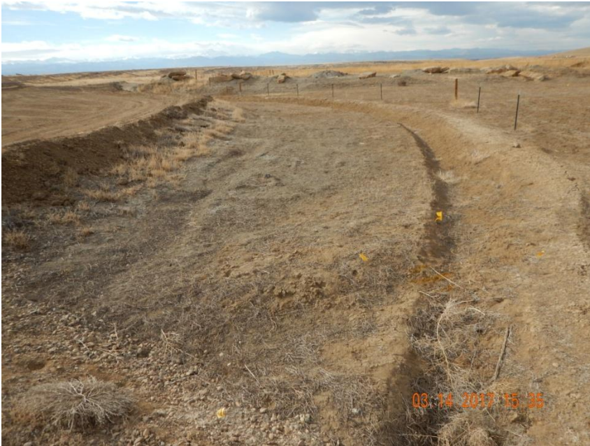
Photo 3. Photo taken from the northeastern location, facing Northwest. A ditch and berm BMP has been installed around the perimeter of the location.
