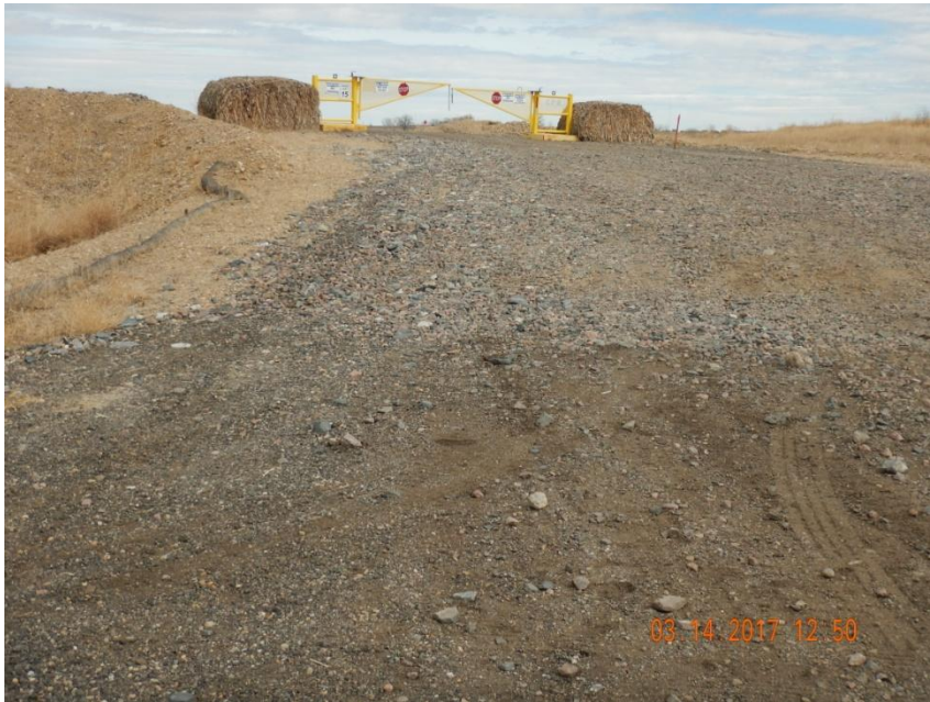
Photo 1. Photo taken from the entrance of location, facing East. Vehicle tracking pad installed.
