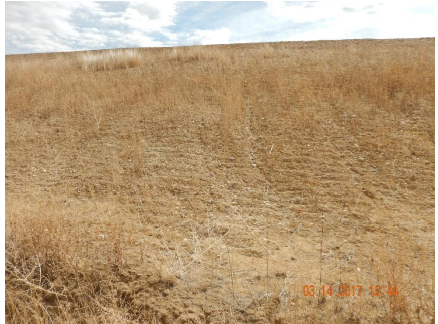
Photo 12. Photo taken from the northern location, facing South. Vegetative growth is sparse along the fill slope so additional stabilization may be required. Appears rill erosion is starting to form throughout portions of the fill slope.
