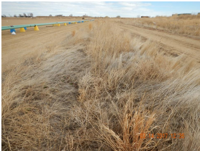
Photo 3. Photo taken from the southern location, facing East. Vegetative growth makes it difficult to observe but a ditch and berm BMP has been installed around the perimeter of the location. Pipeline construction was observed along the eastern, south location area.
