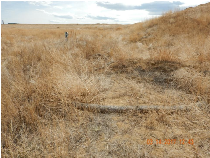
Photo 9. Photo taken from the northeast sediment trap, facing South. Vegetative growth makes it difficult to observe but outlet protection in the form of straw wattles may need maintenance or repair. Wattles do not appear to be properly installed (trenched and backfilled).
