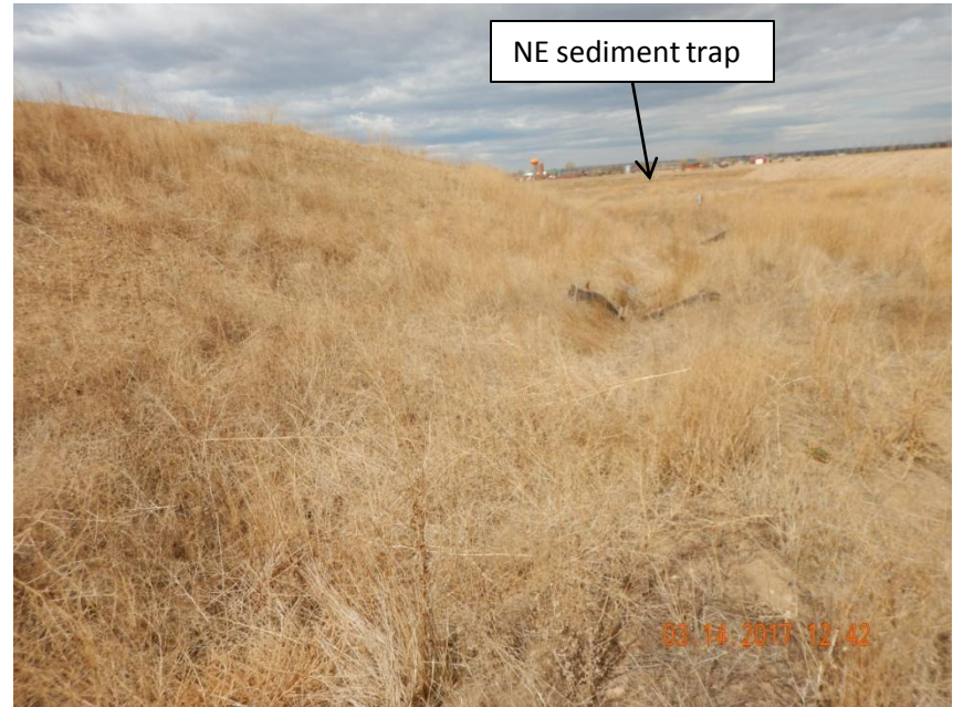
Photo 8. Photo taken from the northeastern location, facing North. Vegetative growth makes it difficult to observe but a ditch and berm BMP has been installed around the perimeter of the location in conjunction with wattles. Fill slope appears to be stabilized along this portion of the location.
