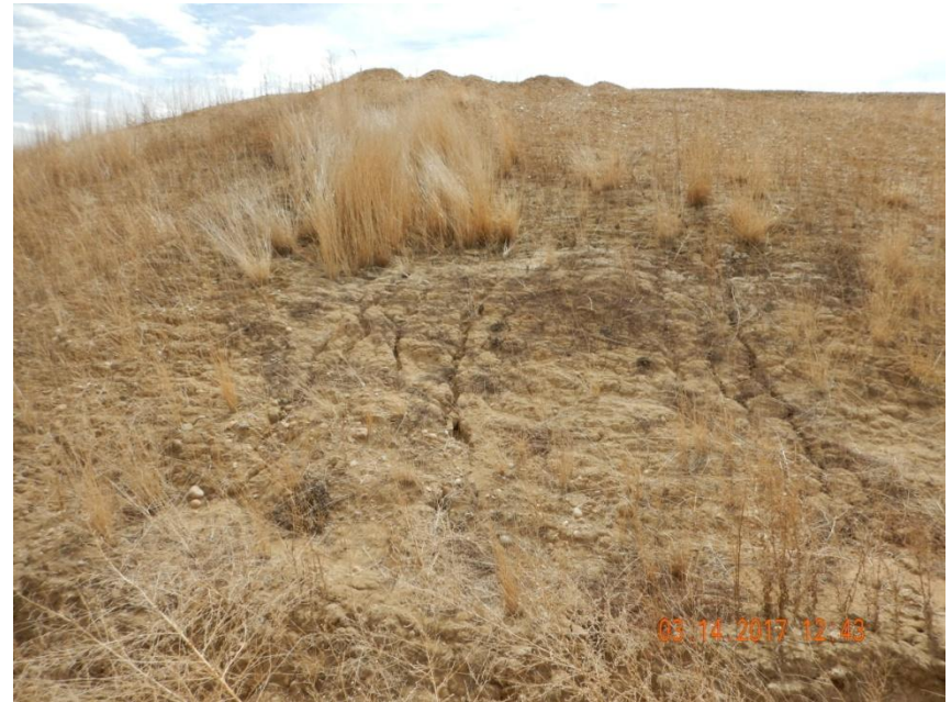
Photo 10. Photo taken from the northeast sediment trap, facing Southwest. Rill erosion occurring along portions of the fill slope. Vegetative growth is sparse so additional stabilization may be required.
