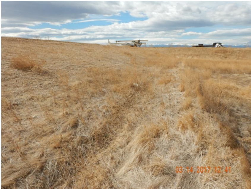
Photo 7. Photo taken from the northeastern location, facing West. Vegetative growth makes it difficult to observe but a ditch and berm BMP has been installed around the perimeter of the location. Fill slope appears to be stabilized along this portion of the location.
