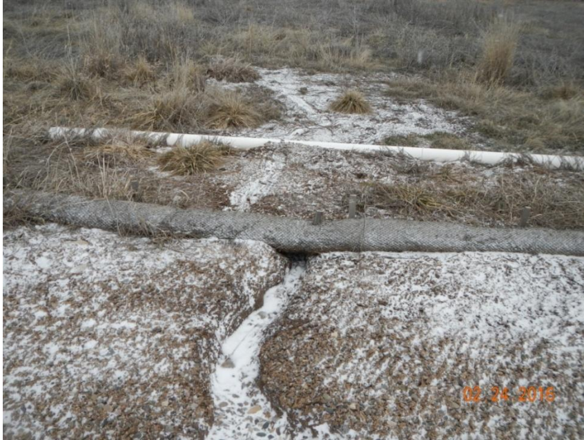
Photo 5: View of erosional channel flowing beneath wattle in the eastern portion of the project area.
