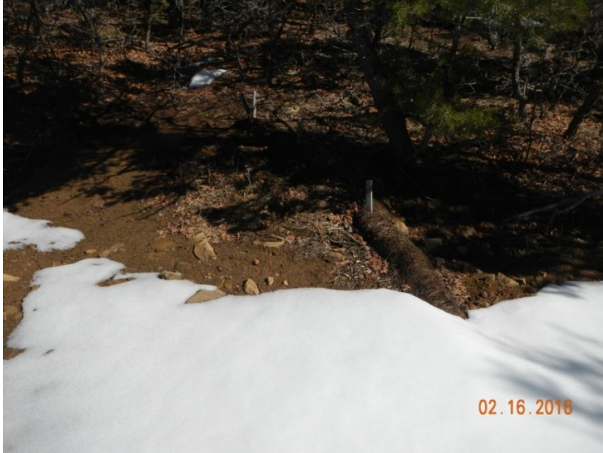
Photo 5: View of stormwater controls that appear to be functioning in the southeastern portion of the project area.
