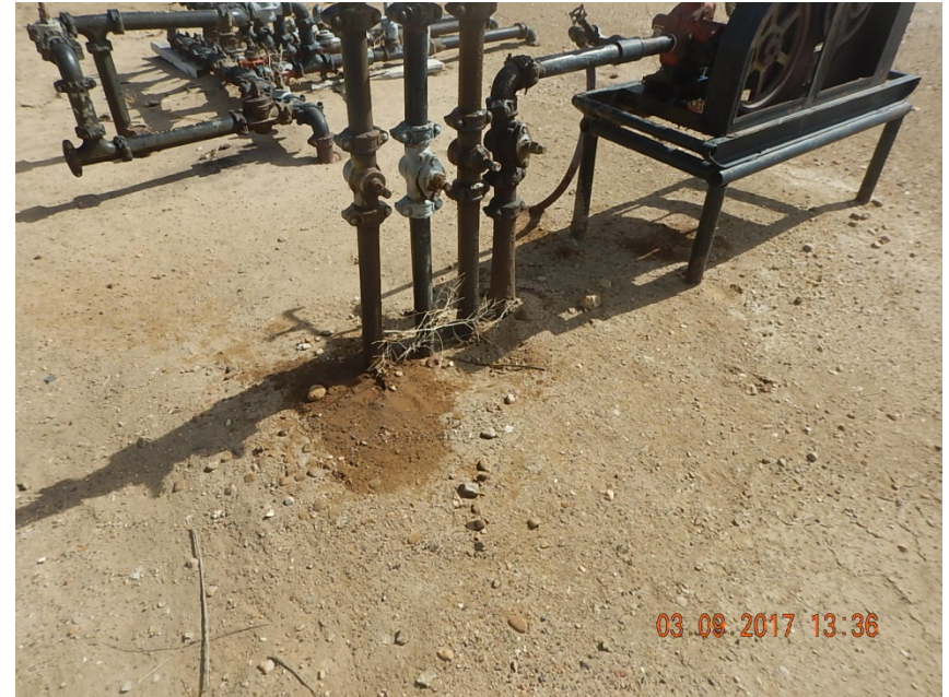
Photo 3: Stained soil at manifold
