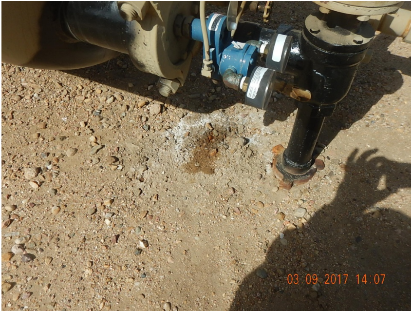
Photo 6: Stained soil and leak at separator
