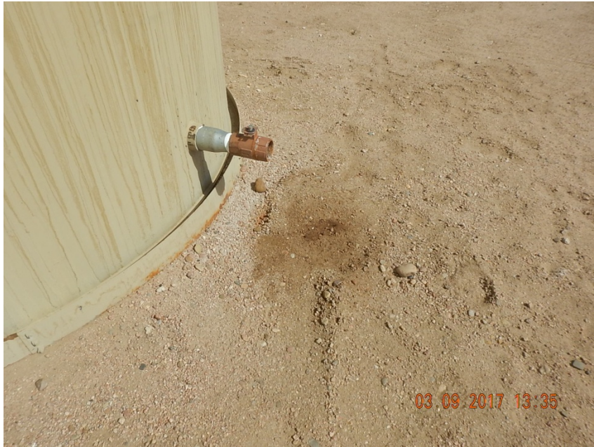
Photo 2: Stained soil at produced water loadout
