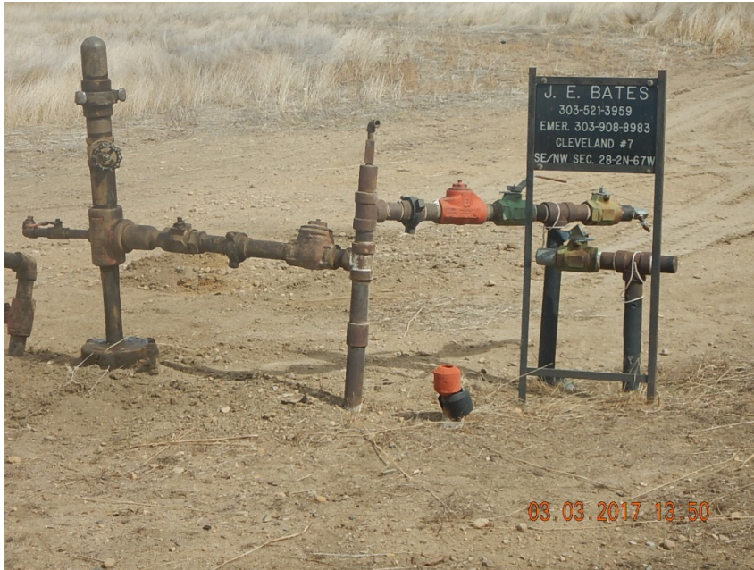
Photo 1: Wellhead, looking E
