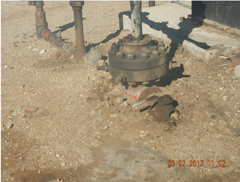
Photo 1: Stained soil at wellhead, no bradenhead
