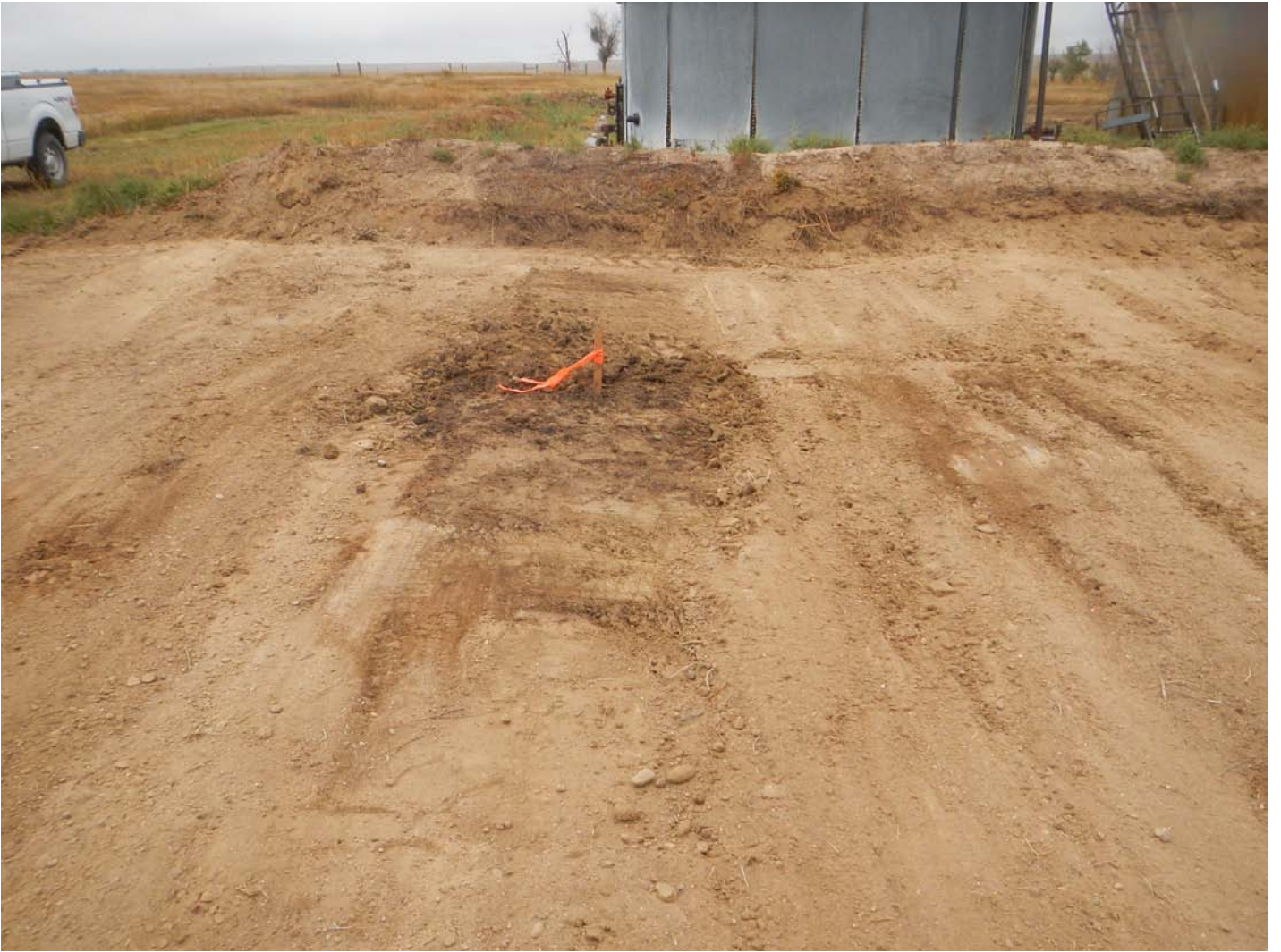
September 21, 2016 view north at Spill ID #447951 area after the impacted soil had been scraped up and included with the Spill ID #446079 soil stockpile.
