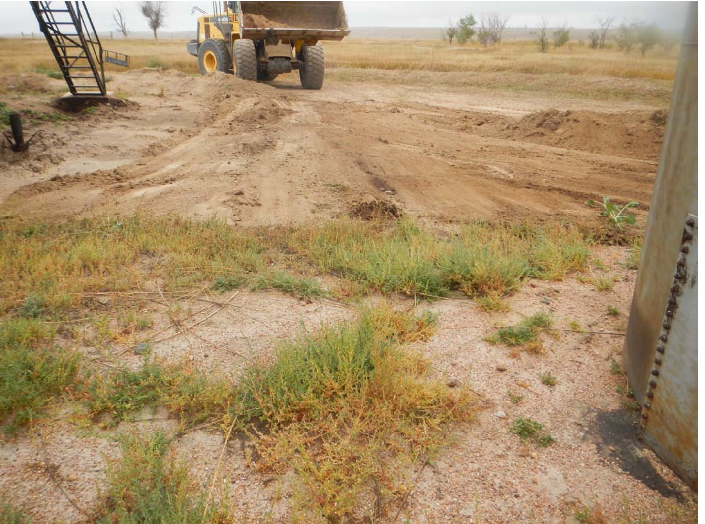
September 22, 2016 view north at the former impacted soil stockpile area and secondary containment reconstruction.
