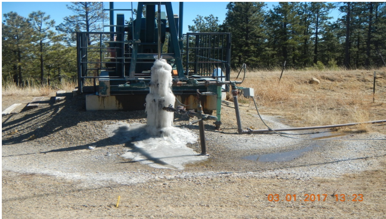
photo 2: There is a water leak which is iced over at the well head.
