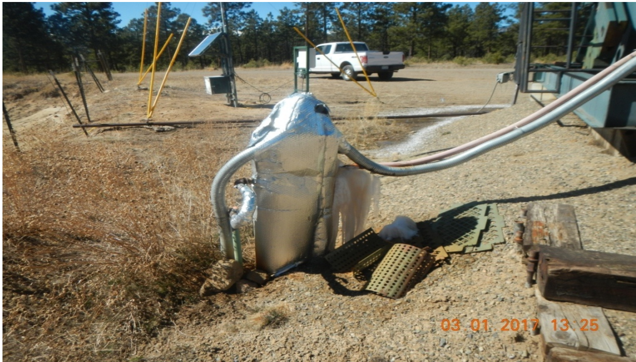
photo 3: Ice was noticed around the insulated piping.
