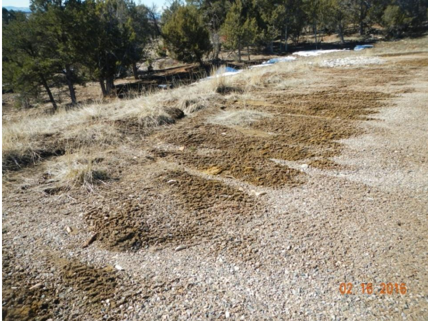
Photo 5: View of rills along the southern edge of the working area where concentrated stormwater flows into the interim reclamation area.
