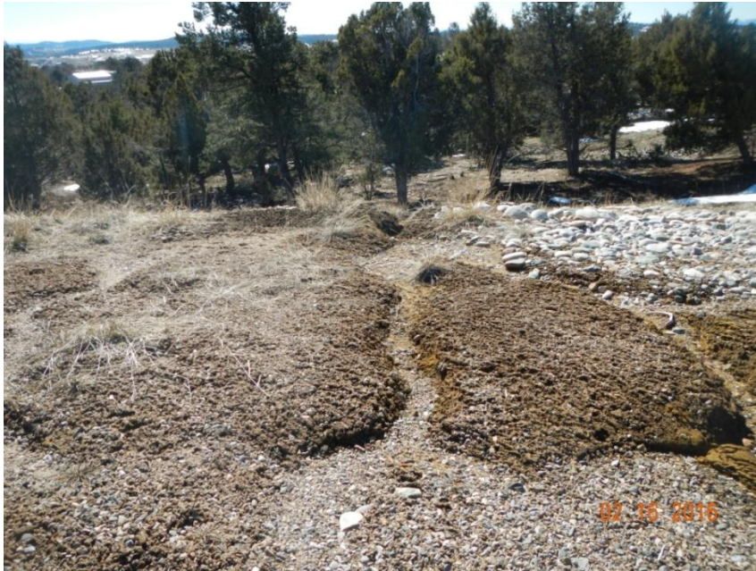
Photo 7: View of erosional controls eroding the southwestern portion of the interim reclamation area.
