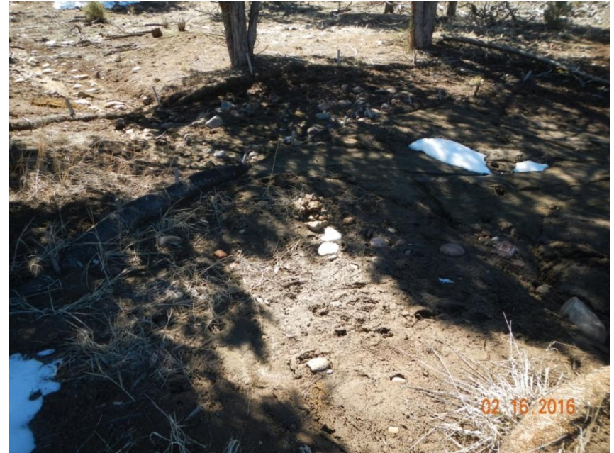
Photo 8: View of wattles along the southern edge of the project area that are full of sediment and no longer functioning.
