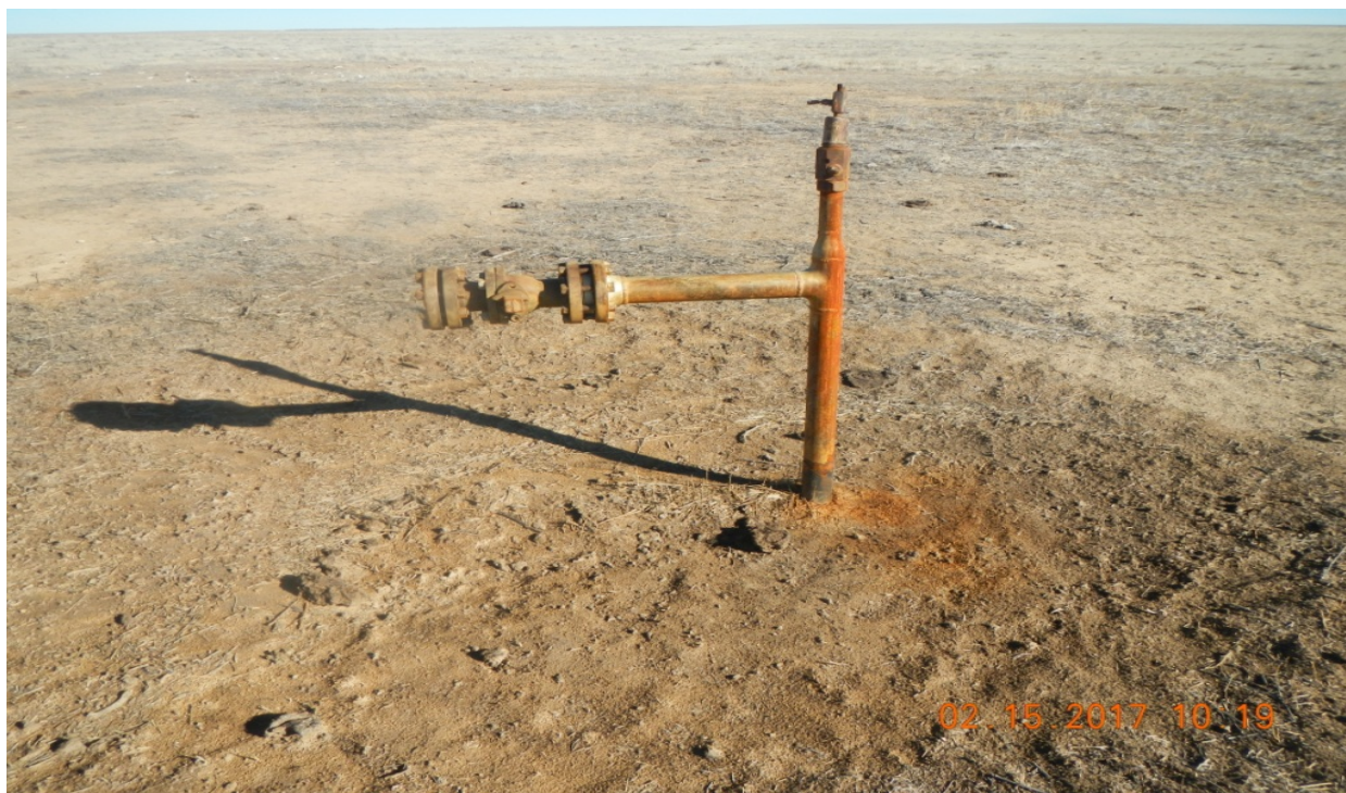
photo 2: Pipe riser remains at the location.
